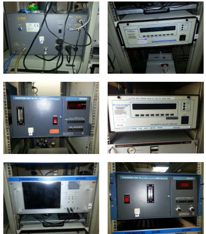
Fig. 2. Equipments used from each monitoring station
