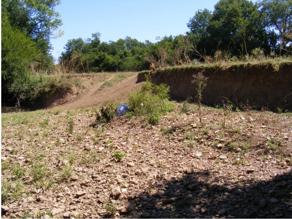
Photo 17. Utility Easement and Cattle Entrance Reach (600 ft) looking at the cattle entrance and left bank erosion.
