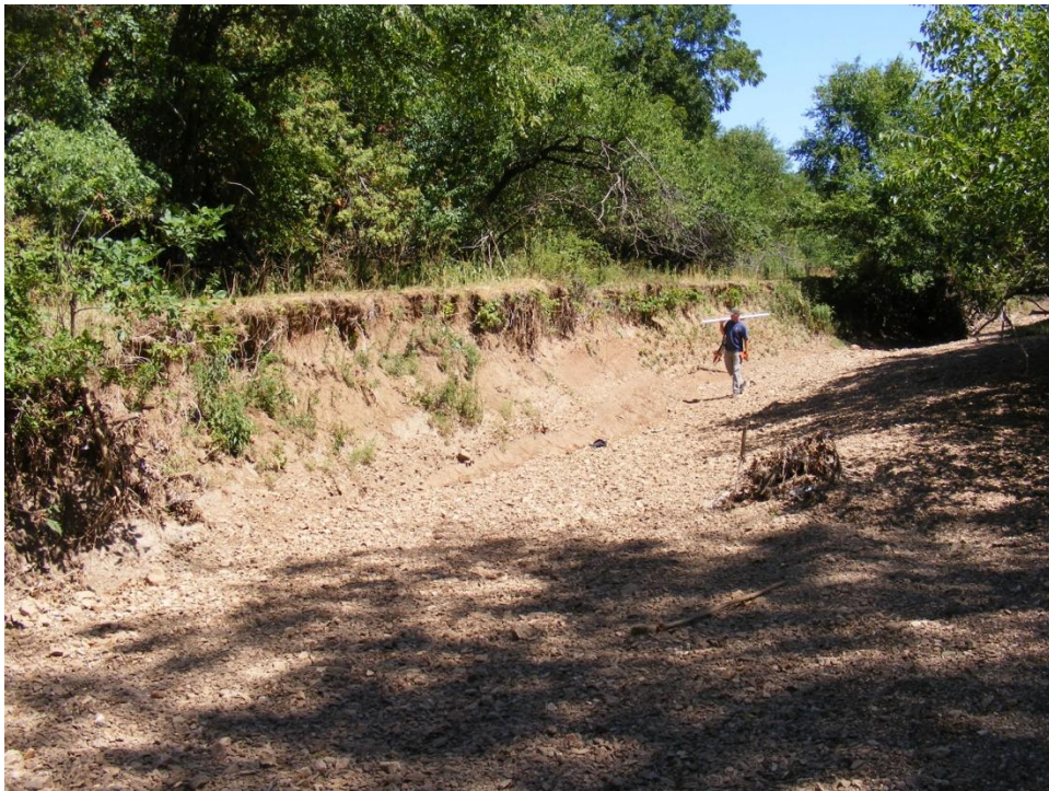
Photo 14. Bank Erosion Reach (1,300 ft) looking at the right bank.
