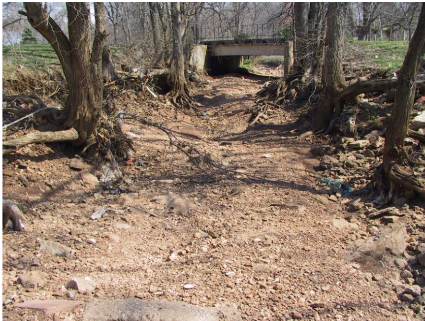
Photo 4. Scour hole at station 2,100 feet
