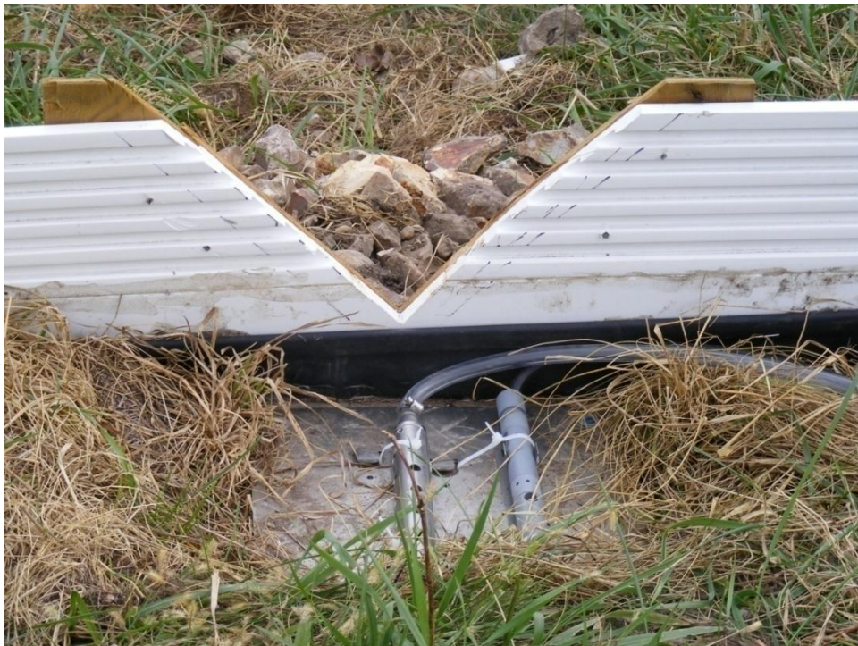
Photo 2. Pressure Transducer and Strainer Location
