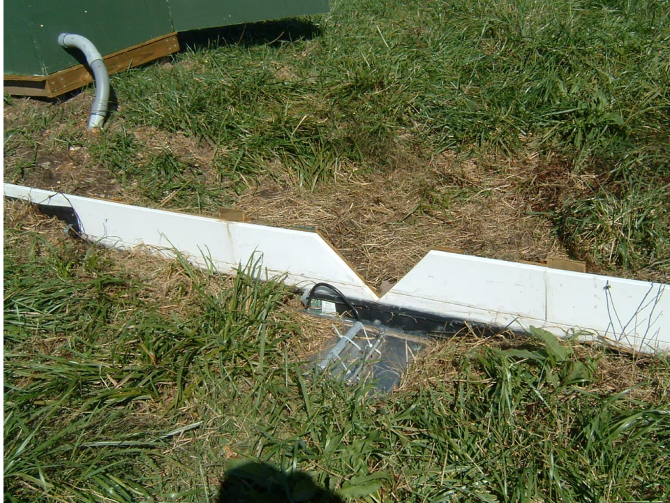
Photo 1. V-Notch Weir, Pressure Transducer, and Strainer Location
