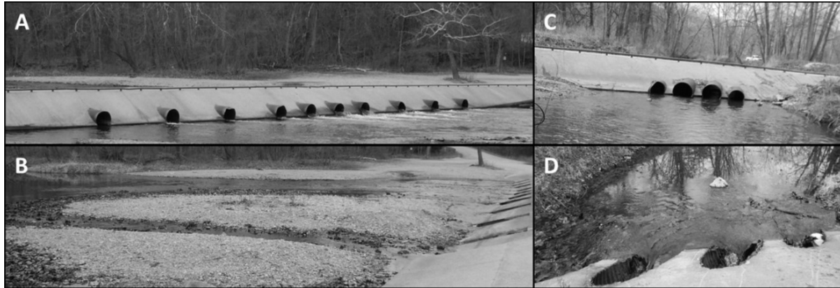
Figure 2. (A) Downstream view of the main channel crossing at Cedar Grove. (B) Upstream view of the main channel crossing showing extensive sediment deposition. (C) Downstream view of the side channel crossing at Cedar Grove. (D) Upstream view of the side channel crossing showing lighter sediment deposition. Photos were taken 9 February 2018. Discharge at the Cedar Grove low-water crossing was 2.33 \text{ m}^3/\text{s} .
