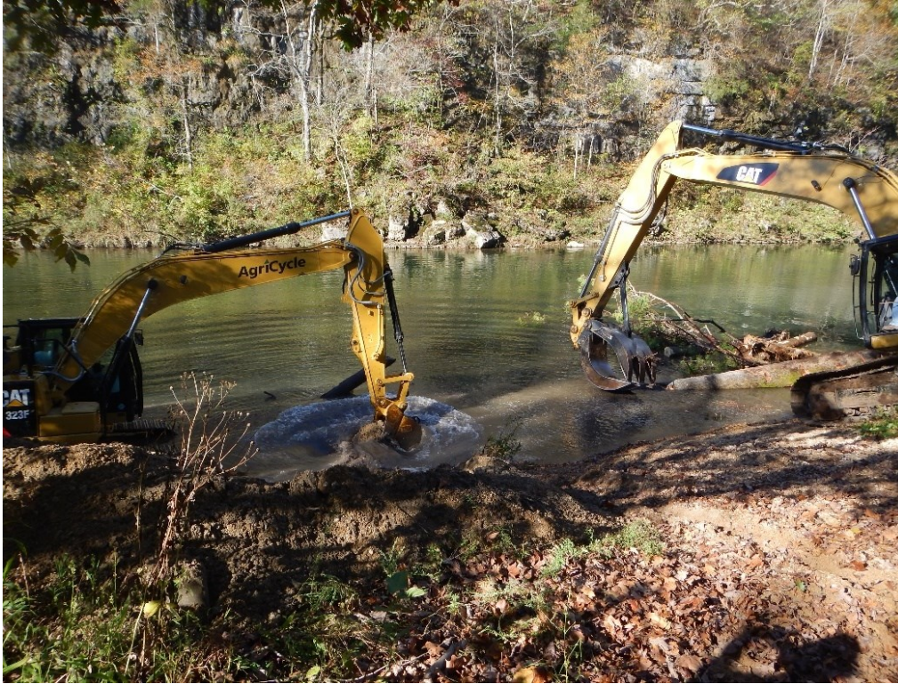
Figure 5. Construction of ELS 1. Excavator digging a trench in the bed for key piece placement.
