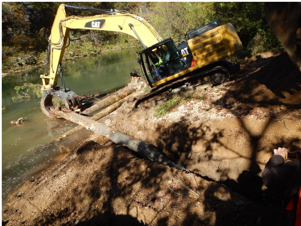
Figure 6. Excavator placing logs in a trench perpendicular to flow positioned over key pieces.
