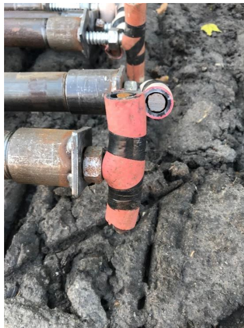
Figure 52. Protective rubber at the ends of the pipes used in McDonough Bridge.
