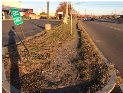
Lack of sidewalk.JPG
