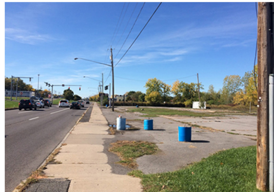
Poor condition sidewalk, no street trees, exposure to sun
