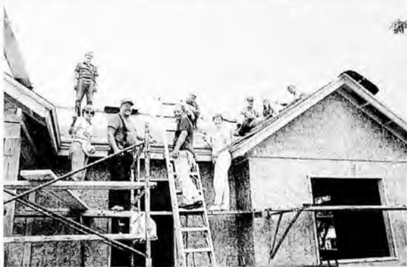
August 6: Bud Nichols and his crew of volunteers take a photo break from their roofing activities.
