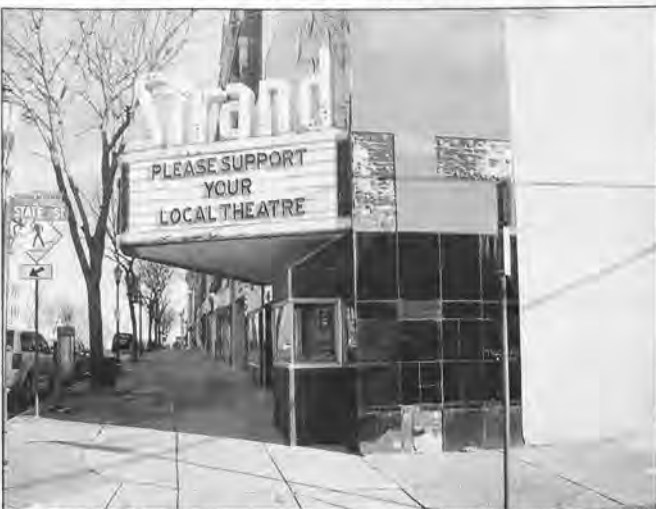
Looking north on Main Street, the art deco facade of the historic Strand Theatre shows 2' x 2' tiles missing and rust on the marquee after 64 years of exposure to the elements. Photo by Doug Hickerson.
