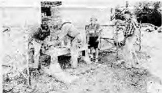
August 13: Bud Nichols gives some advice to Jim Bolthouse on how best to trim the edge of the porch landing.
