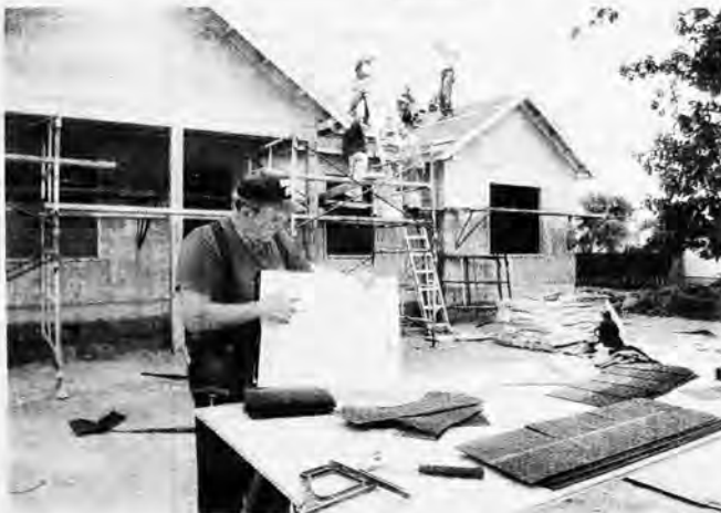
August 6, 1998. Bud Nichols, Brockport Habitat for Humanity project manager, points out the plan for the Brockport Habitat home in front of a busy crew of volunteers "scaling new heights." Above, Nichols does some nail sorting in addition to being the guide and inspiration for a host of volunteers. His savvy and patience has helped train the volunteers and resulted in quality work being done on the project. A photo essay inside shows the progress on the site over several weeks. Photographs for Westside News Inc. by Walter Horylev.
