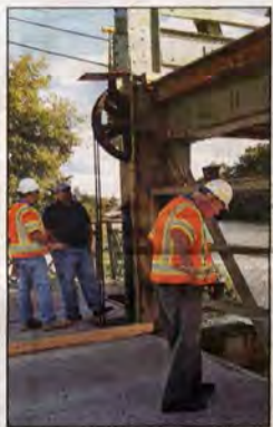
Lift bridge inspection includes examination of pulleys, cables, gears and other mechanism with the bridge raised. Photo by Dianne Hickerson.
