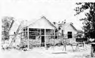
August 6: An overview of the Habitat House as of this date. Construction began late in April; it should be finished sometime around Thanksgiving.
