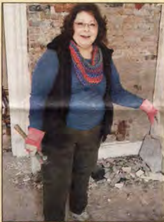
Carol Hannan stops for a photo while removing plaster from a chimney in the 52 State Street house she is renovating. She uses other more creative skills, sometimes with volunteers, to return many deteriorating Brockport houses to family homes. Her goal is to "revitalize Brockport house by house." Photo by Dianne Hickerson.
