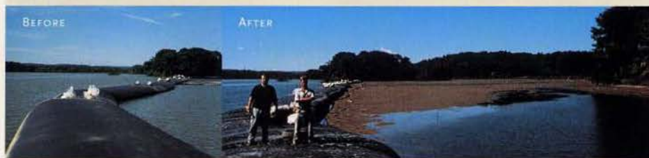
BEFORE AND AFTER DEWATERING USING AQUA DAMS IN COOTES PARADISE IN HAMILTON, ONTARIO, CANADA.
