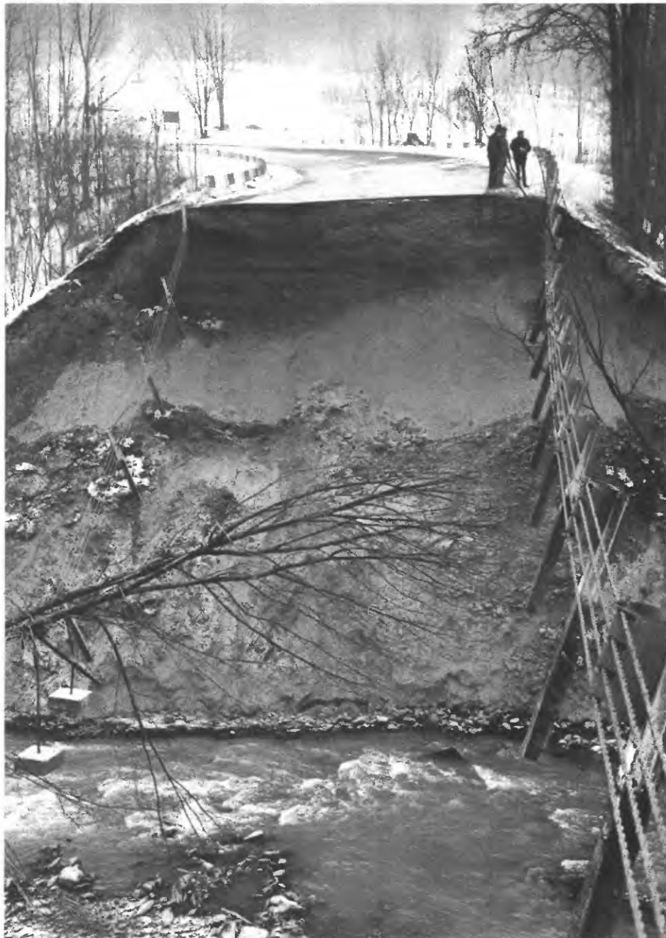
Figure 9A. Washout on Chase Brook Road across Chase Brook near Cannonsville Reservoir in Delaware County, N.Y., January 19, 1996. (Photograph courtesy of the Walton Reporter, January 24, 1996, p. 6.)
