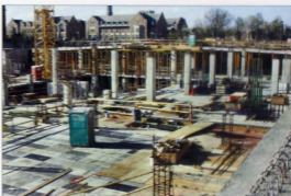
But by April, the parking garage under the new University Center begins to take shape.
