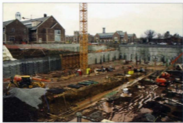
In November, the former home of Price Hall was still just a gaping, muddy hole.
