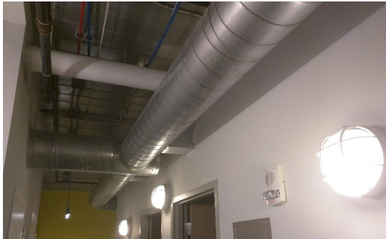
Fig. 4 Ceiling-suspended ducts in suite 117
