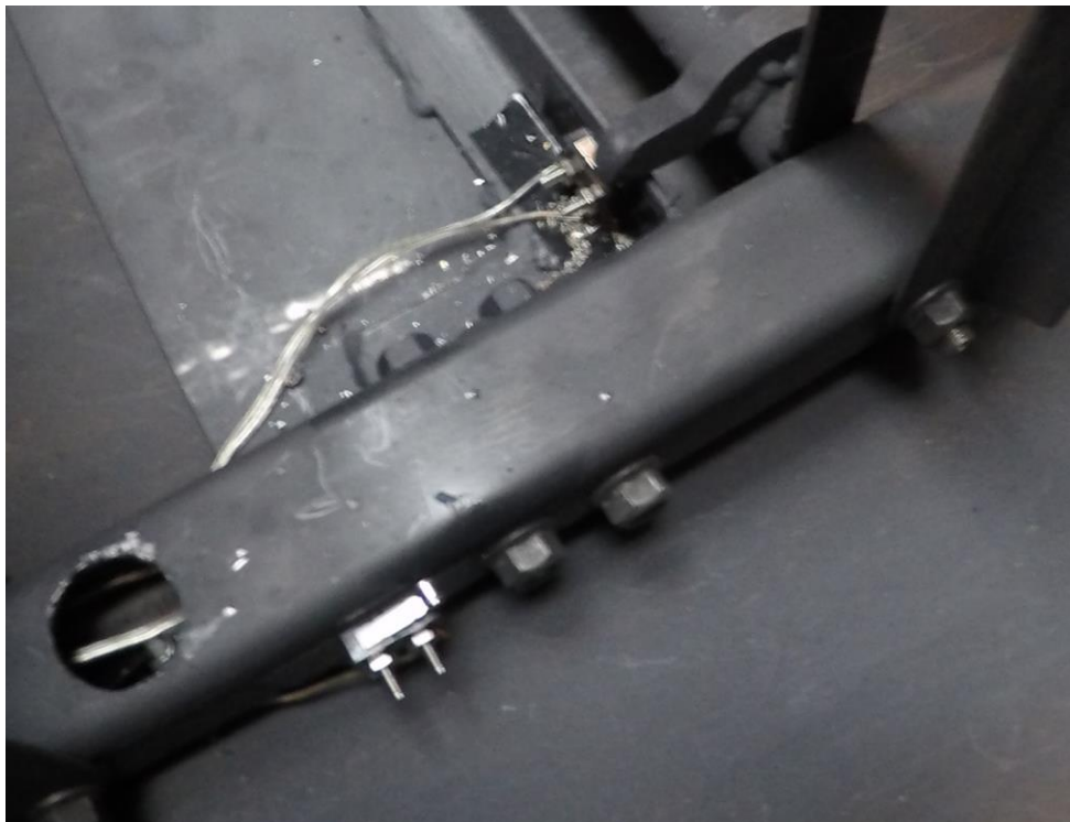
Figure 15 - TLA Limit Switches
