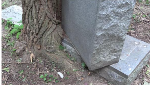
Figure 3.1 Broken Headstone at WPC. (Denise Ward Brown Personal Collection, 2016, JPEG.)
