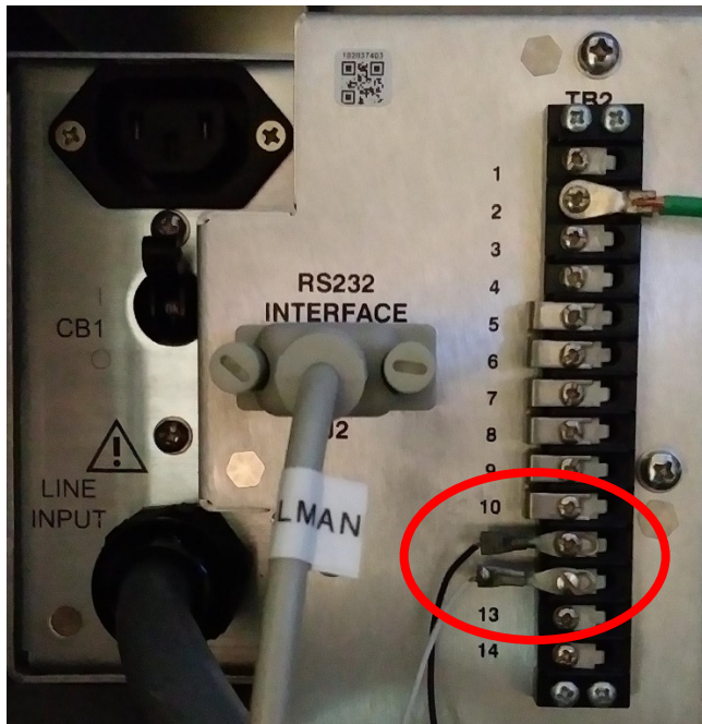
Figure 5.9 Hardware interlock input on the back of the Spellman power supply.
