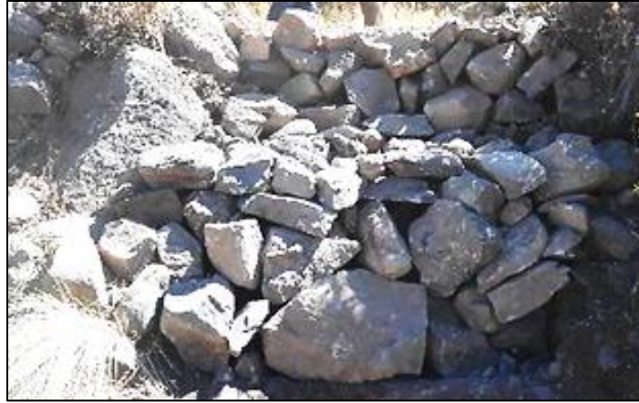
Figure 8.3: Photos of stacked stone riser wall. Note the unworked stone that are irregularly stacked in various orientations.
