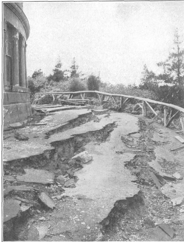
B. SLIP OF FOUNDATION OF CYCLORAMA, STRAWBERRY HILL, GOLDEN GATE PARK, SAN FRANCISCO, CAUSING COLLAPSE OF THE STRUCTURE.
