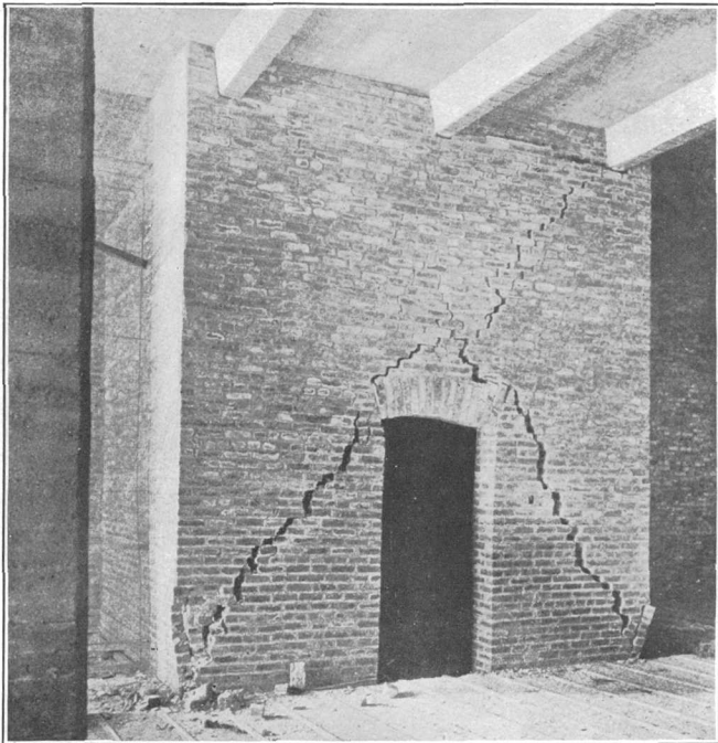
A. EARTHQUAKE CRACKS IN WALL OF VAULT, CALIFORNIA CASKET COMPANY'S BUILDING, SAN FRANCISCO.
