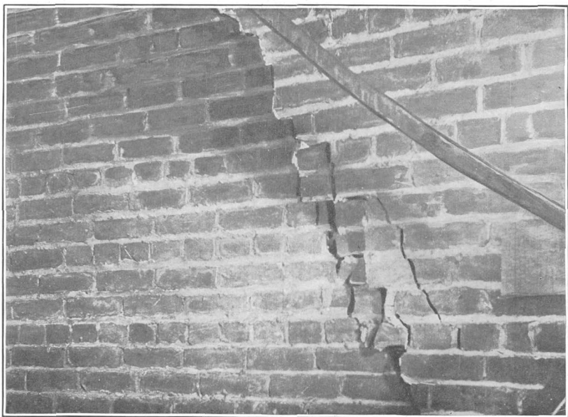
B. EFFECT OF SEVERE SHAKING ON WELL-BONDED BRICKWORK FILLED WITH GOOD MORTAR, TOWER OF UNION FERRY BUILDING.
