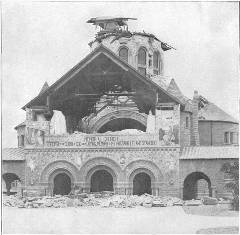
B. COLLAPSED TOWER AND GENERAL EARTHQUAKE WRECKAGE, MEMORIAL CHURCH, LELAND STANFORD JUNIOR UNIVERSITY.
