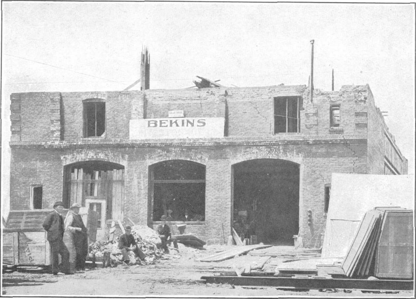
A. EARTHQUAKE ENDURANCE OF REENFORCED-CONCRETE BUILDING, BEKINS VAN AND STORAGE COMPANY'S WAREHOUSE, SAN FRANCISCO, UNDER CONSTRUCTION.
