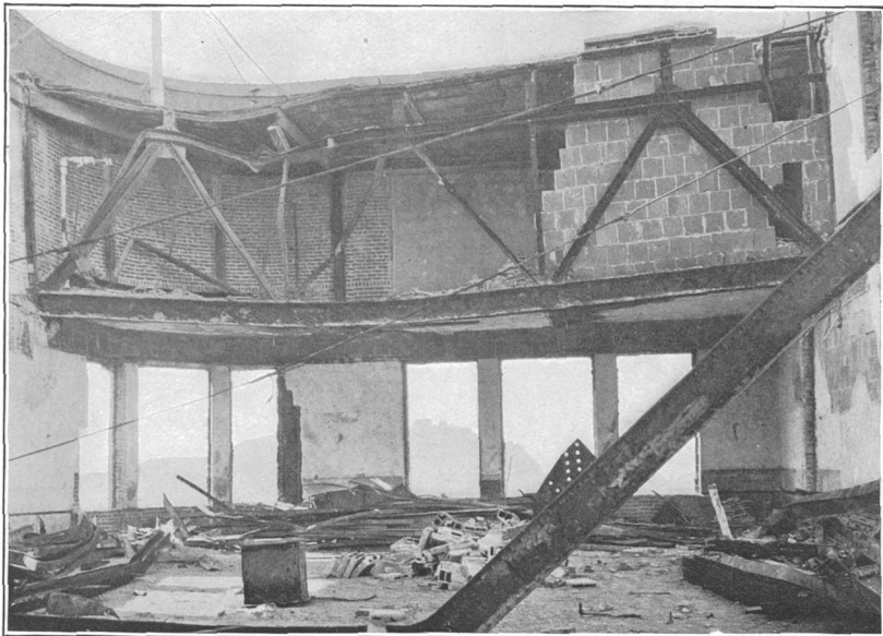
A. ROOF TRUSSES DAMAGED BY HEAT, THROUGH FAILURE OF TERRA-COTTA COVERING, MUTUAL LIFE BUILDING, SAN FRANCISCO.
