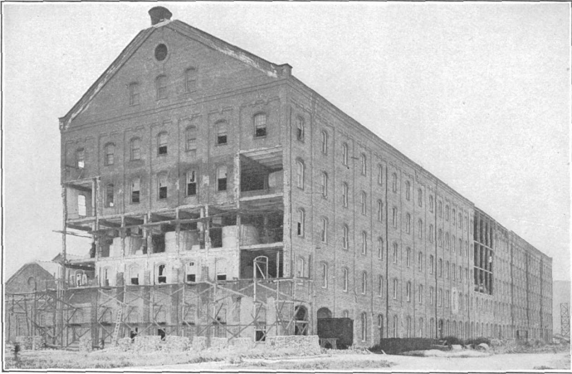
A. EFFECT OF EARTHQUAKE ON THE END AND THE INSUFFICIENTLY BRACED CENTRAL PORTION OF A BRICK BUILDING, SPRECKELS'S SUGAR MILL, ABOUT 4 MILES SOUTH OF SALINAS.
