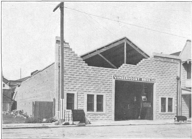
B. WALL THROWN DOWN BY EARTHQUAKE VIBRATIONS OF ROOF TRUSSES WHICH WERE NOT TIED TO WALL, VANDERVOORT BROTHERS' LIVERY, PALO ALTO.
