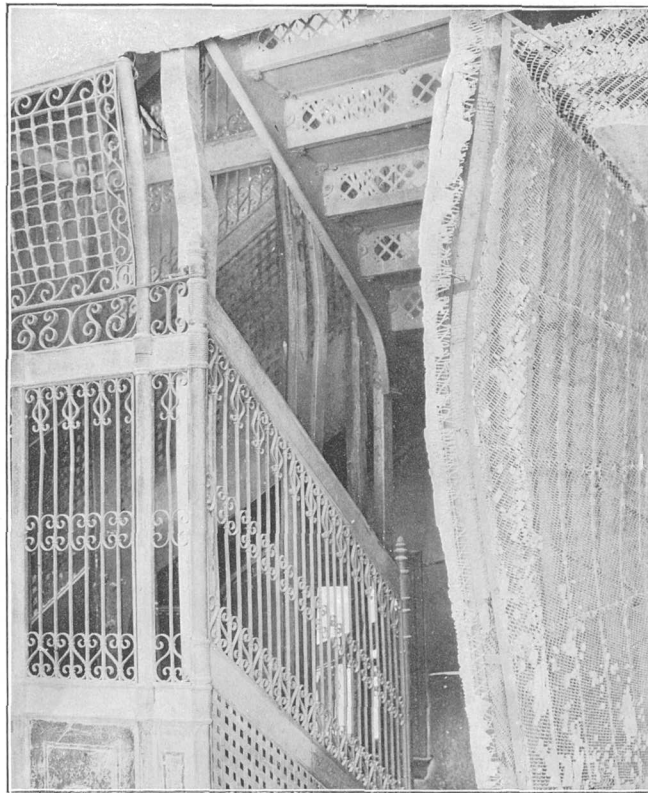
B. WARPING OF PLASTERED METAL-LATH COVERING BY FIRE, MURPHY BUILDING, SAN FRANCISCO.
