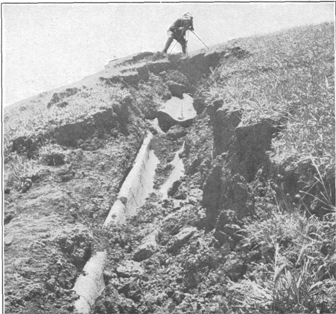
A. COLLAPSED PILARCITOS 30-INCH WROUGHT-IRON PIPE LINE, NEAR TRESTLE CROSSING THE FAULT.
