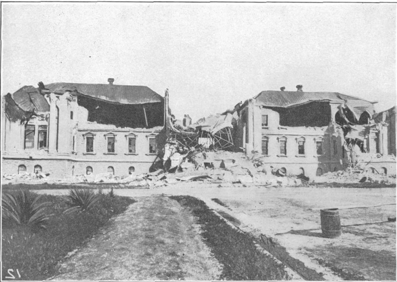
B. COLLAPSE OF BRICK WALLS, CAUSING DESTRUCTION OF STEEL SKELETON DOME OF GYMNASIUM.
