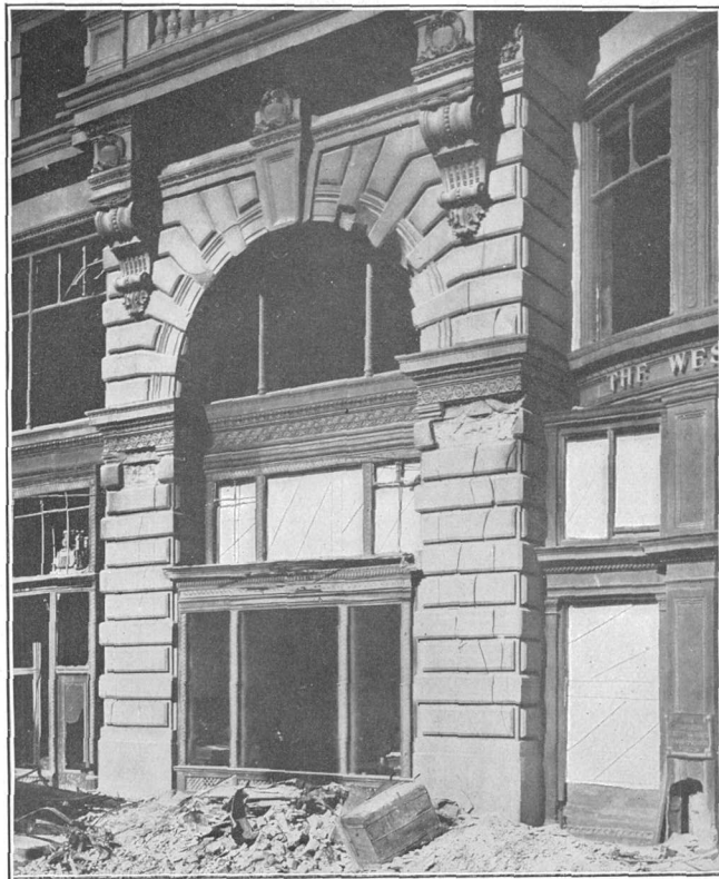
B. EARTHQUAKE DAMAGE TO STONE PIERS, JAMES FLOOD BUILDING, SAN FRANCISCO.
