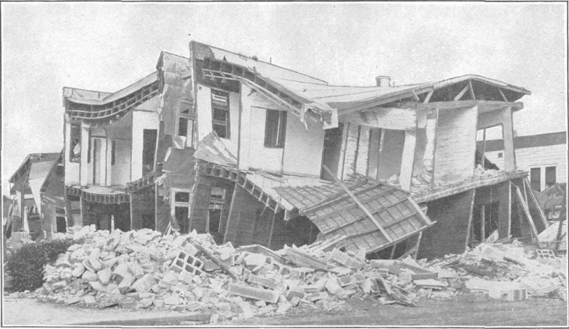
A. COLLAPSE DUE TO LACK OF TIE BETWEEN WALLS AND FRAME, THIELE BUILDING (CEMENT BLOCK), PALO ALTO.
