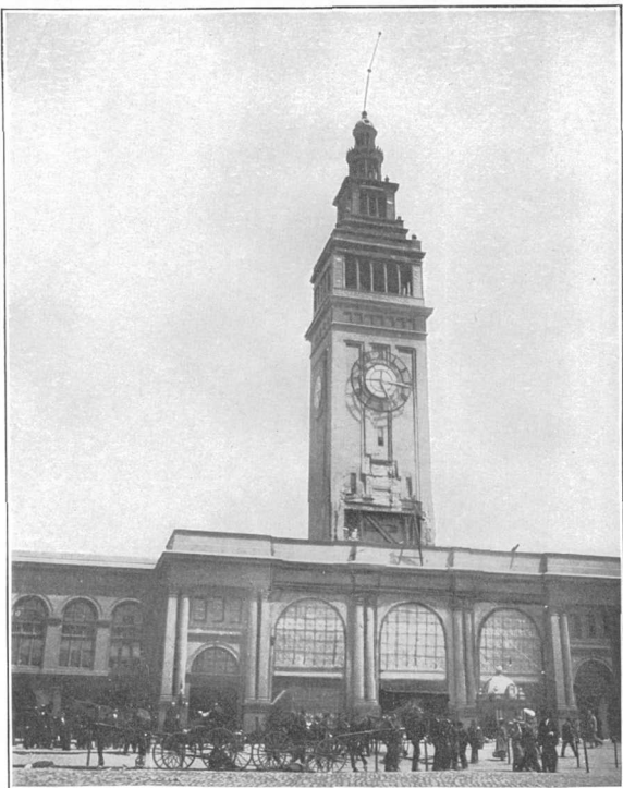
A. BRICKWORK THROWN DOWN BY EARTHQUAKE VIBRATION, TOWER OF UNION FERRY BUILDING, SAN FRANCISCO.
