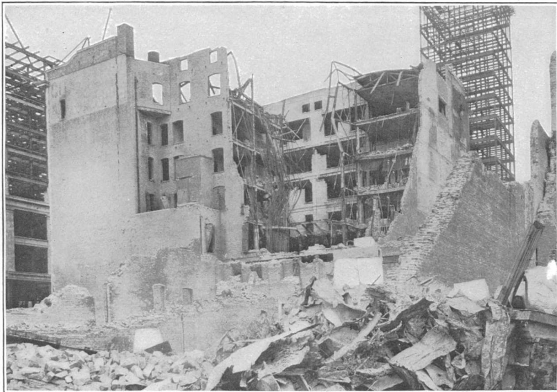
A. COLLAPSE OF BUILDING DUE TO BUCKLING OF COLUMNS, SPRING VALLEY WATER COMPANY'S BUILDING, SAN FRANCISCO.
