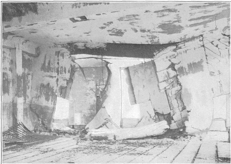
B. FAILURE OF SUSPENDED CEILING, HALL OF JUSTICE, SAN FRANCISCO.
