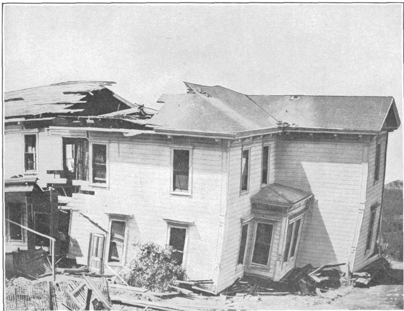
B. HOUSE ON LINE OF FAULT, TORN ASUNDER BY EARTHQUAKE.
