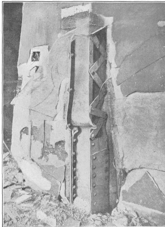
B. BUCKLING OF COLUMNS DUE TO FAILURE OF WIRE-MESH-AND-PLASTER FIREPROOFING, HOTEL HAMILTON, SAN FRANCISCO.
