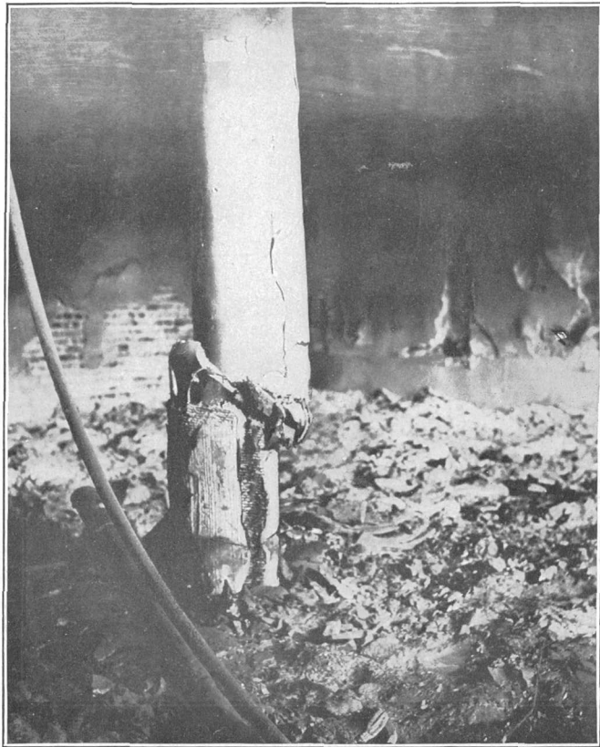
A. FAILURE OF BASEMENT COLUMN DUE TO FIRE, SLOANE BUILDING, SAN FRANCISCO.
