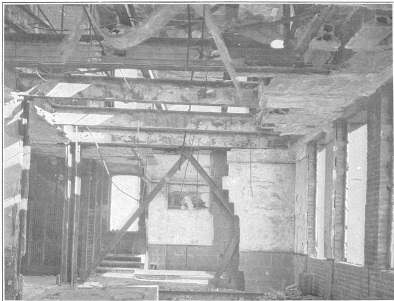
B. FAILURE OF TERRA-COTTA TILE COVERING IN FIRE, UNION TRUST COMPANY'S BUILDING, SAN FRANCISCO.
