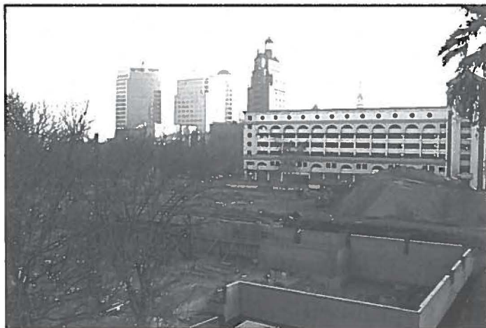
At the downtown Sacramento site of the future Cal/EPA headquarters, the foundation and basement walls are starting to outline the footprint of the 950,000 square foot structure.
