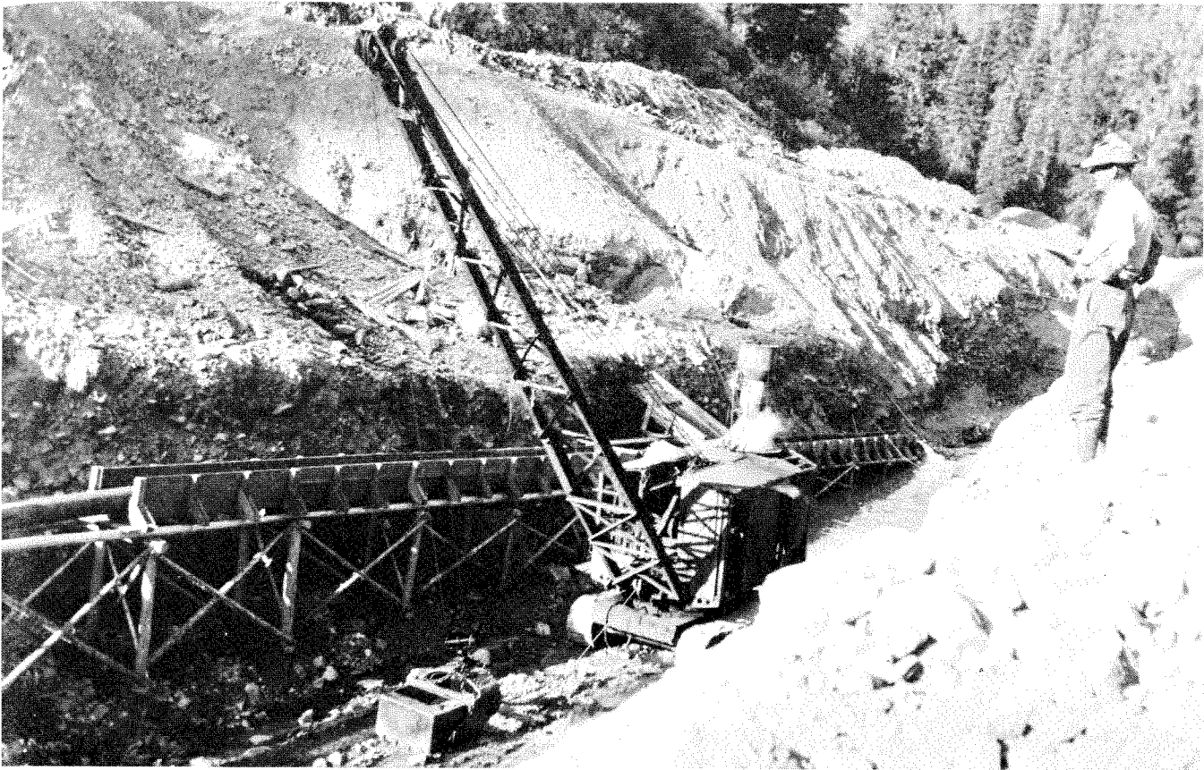
Photo 70. Steam Dragline Operation, Trinity River District. The photo was taken at Coffee Creek, Trinity County, in the 1920s. Photo by C. V. Averill.
