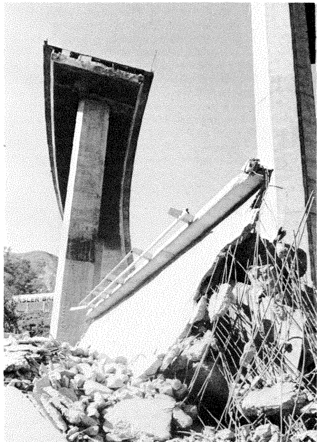
Photo 1. Highway overpasses that collapsed during the San Fernando earthquake of February 9, 1971. Photo courtesy Newhall Signal.
