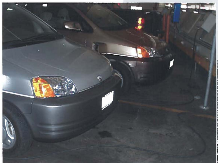
Electric vehicles recharging at California Department of General Services parking facility, Sacramento, California
