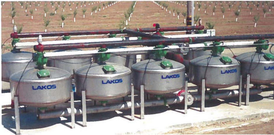
Drip irrigation system protected by sand media filters, Fresno, California
