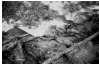
Fig. 9. Perforated hose sprinkler system.
