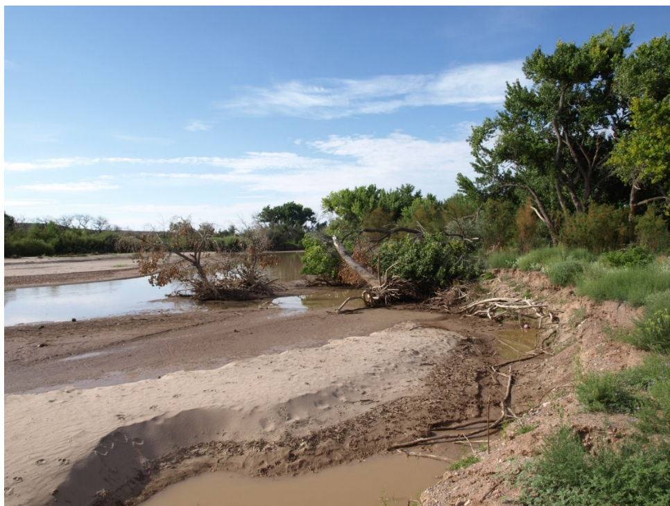
Photo 8: Bank erosion and deposition at Arroyo de las Cañas and Rio Grande confluence (AuBuchon, August 2017)
