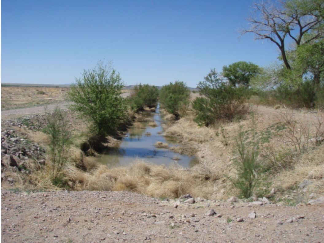
Photo 2: Elmendorf Drain, south branch before maintenance (April 2012, Grogan)
