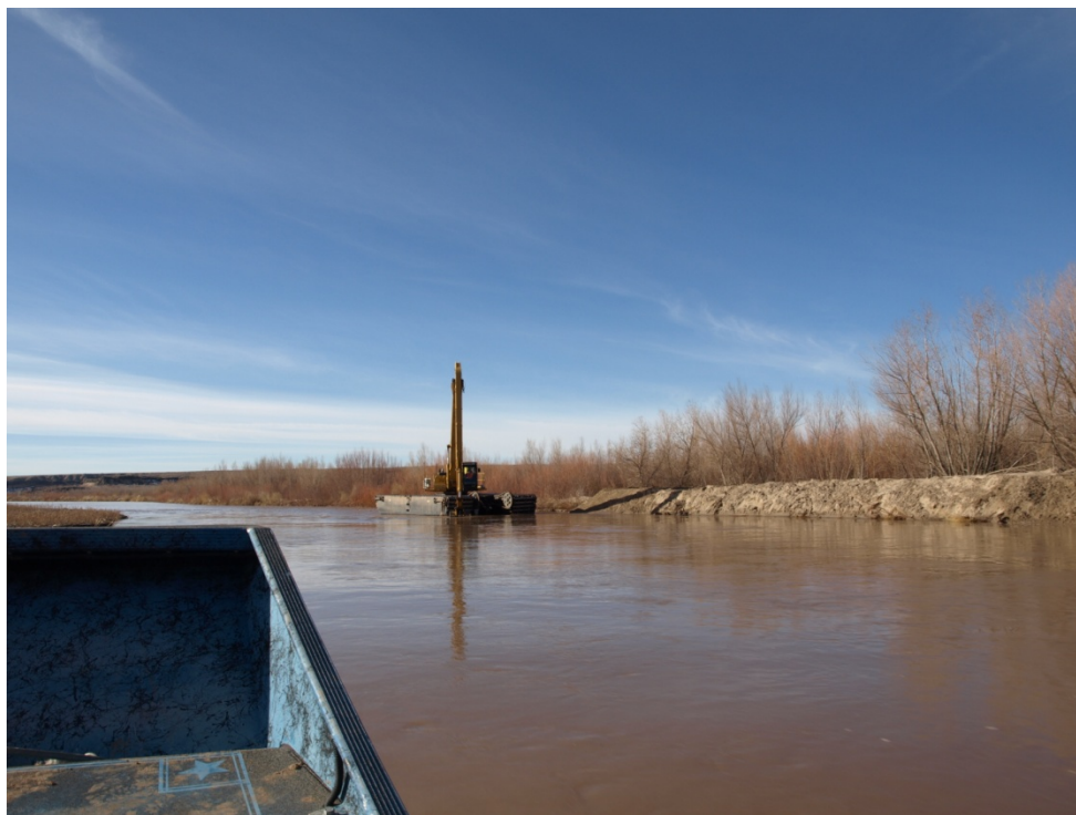
Photo 1: Amphibious excavator working on west berm of the Temporary Channel (January 2012, Casuga)
