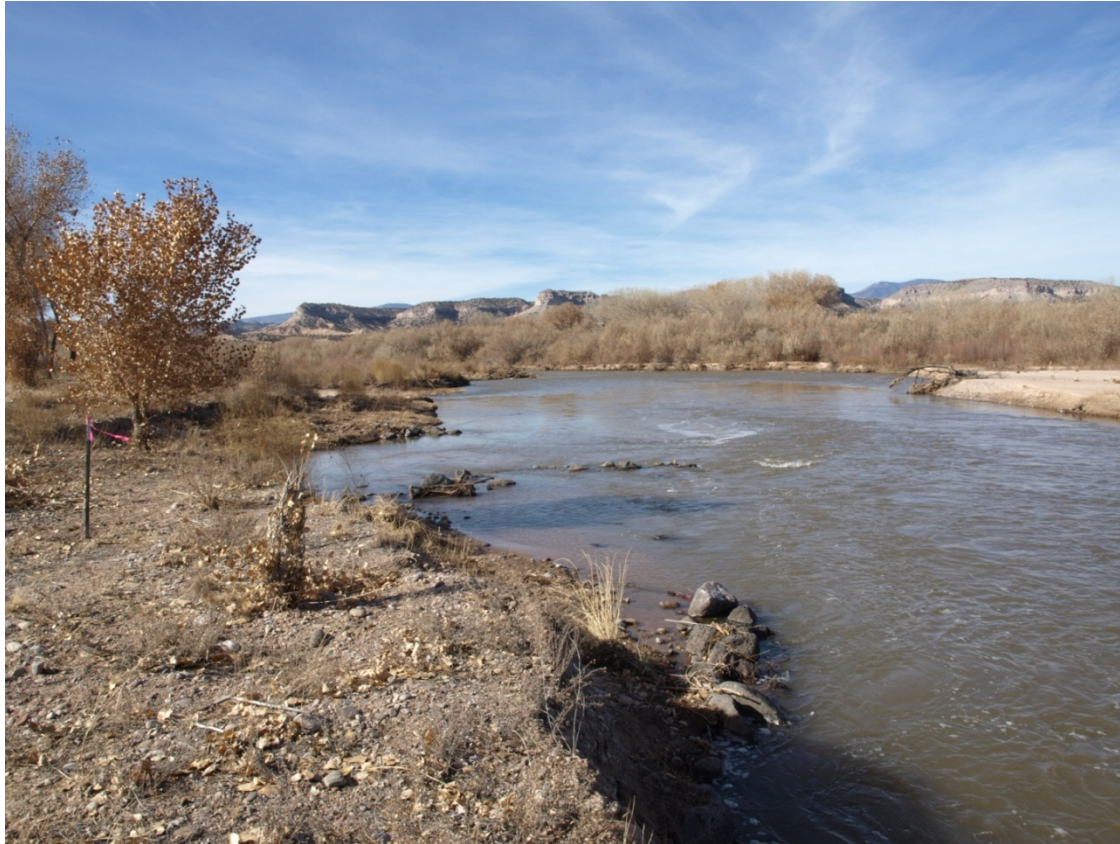
Photo 4: San Ildefonso bankline erosion, showing exposed rock vanes (December 2012, AuBuchon)
