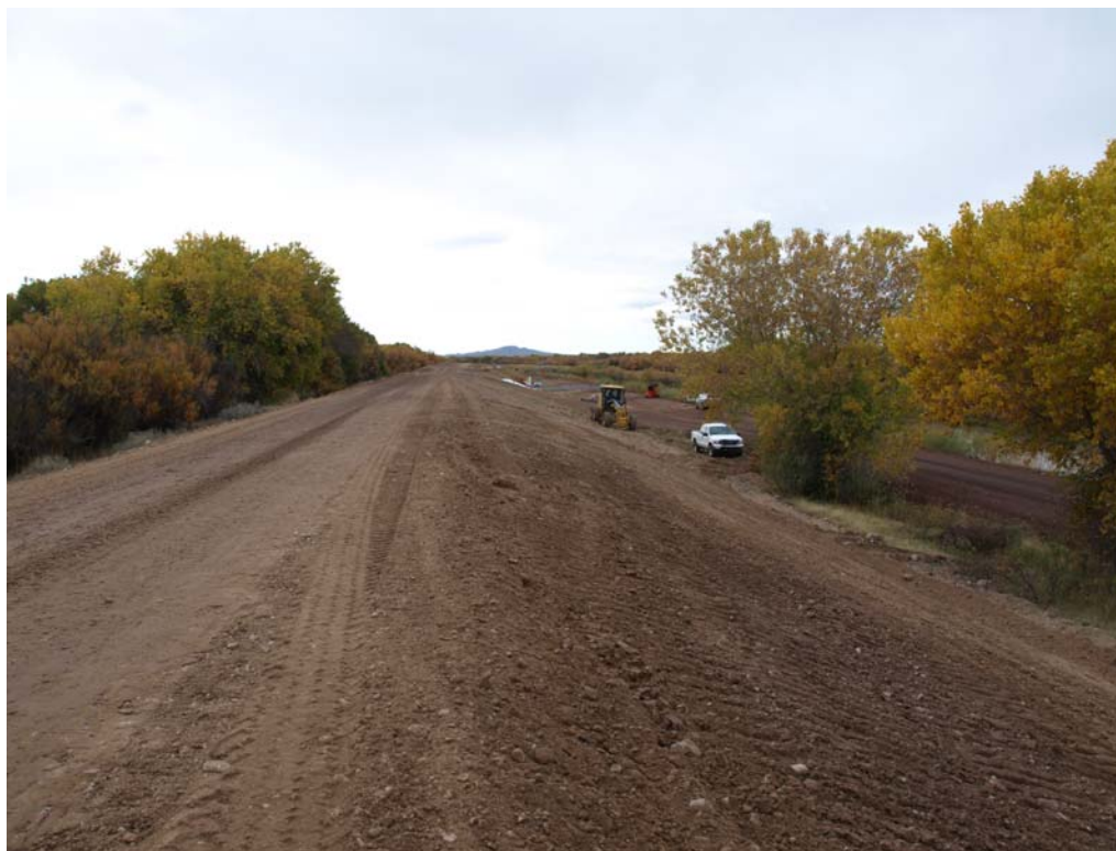
Photo 15: A completed section of the 2009 Bosque del Apache Levee ARRA improvements (October 2009, Rolland)
