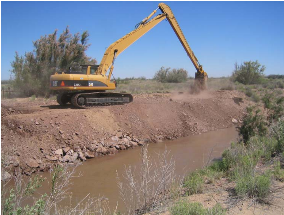
Photo 4: Reclamation construction crews repairing washout at Drain Unit 7 Extension, near the north end of the Ladd Gordon Waterfowl Complex (June 2010, Weems)
