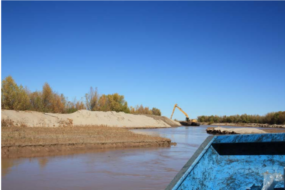
Photo 3: Amphibious excavator working on Breach B south of the Red Rock Staging Area (November 2010, Holste)
