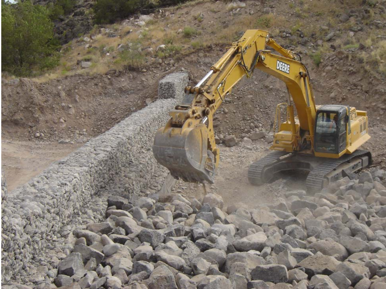
Photo 7: Gabion weir structure at the Salazar Pit, equipment is placing apron material on upstream side of weir (July 2005)
