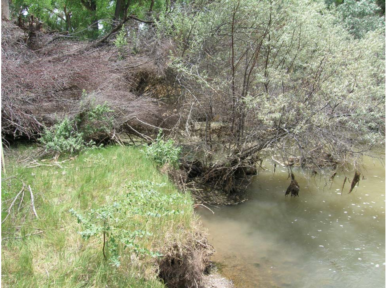
Photo 11: Eroding bankline at River Mile 228.9 on the Pueblo of Cochiti, July 2005
