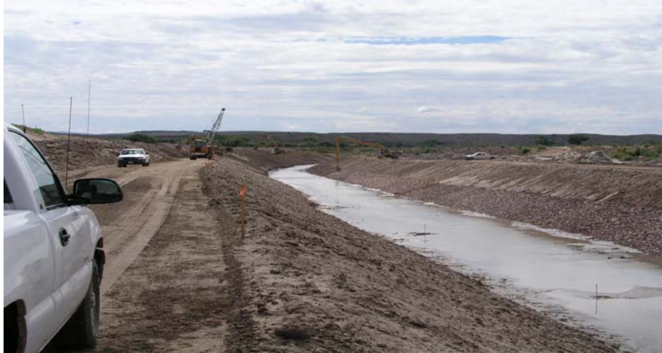
Photo 17: Photo taken on 08-24-05, showing new Low Flow Conveyance Channel section at Station 1895+00 looking downstream. Photo shows completed riprap slope protection on the west side of new conveyance channel. Also shown is a Linkbelt 4300 Excavator performing final slope excavation on the east side of the conveyance channel. Photo taken by Rudy Bernal, Bureau of Reclamation.
