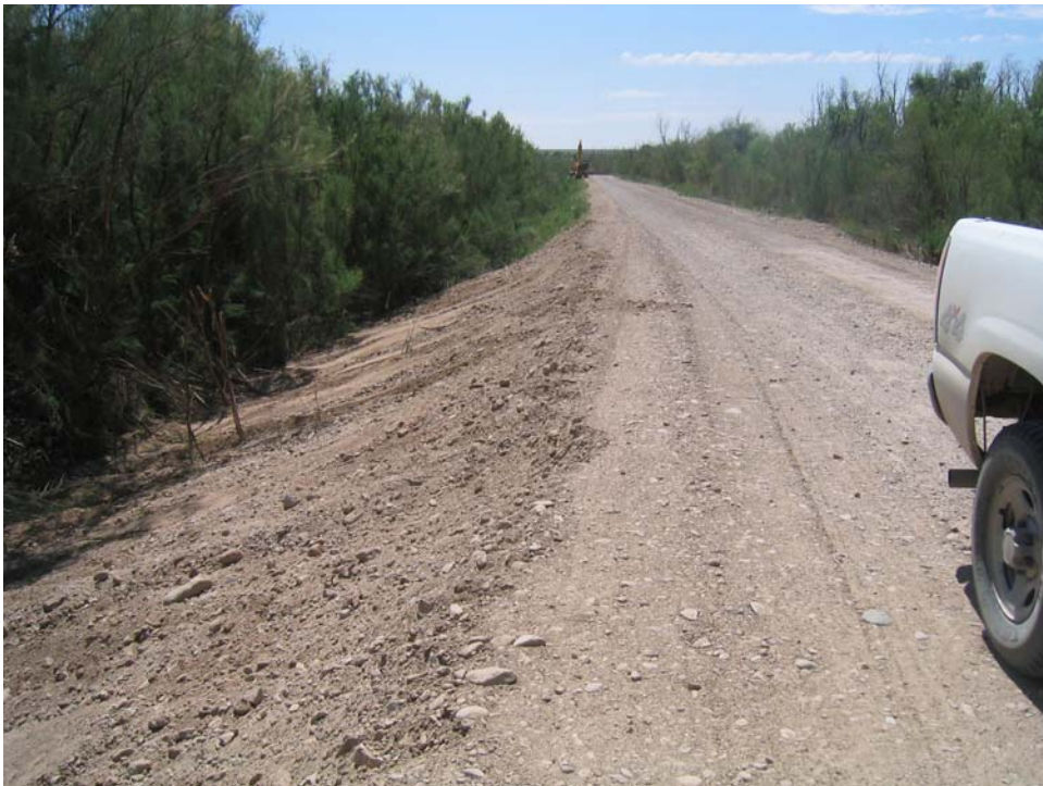
Photo 24: Tiffany Levee showing completed placement of embankment material on the riverside of the Tiffany Levee (2005)
