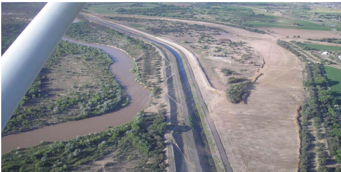
Photo 14: Photo taken 06-10-05, looking south at San Lorenzo Arroyo Settling Basin. Photo shows the area cleared of vegetation for excavation of the realigned Low Flow Conveyance Channel.
