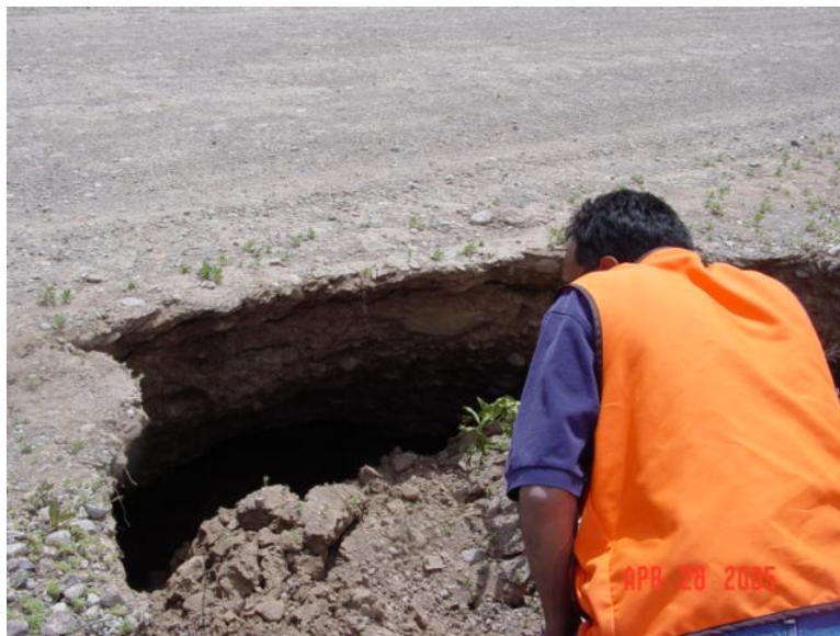
Photo 27: San Marcial Levee near Ft. Craig showing void created by piping through the levee (2005)
