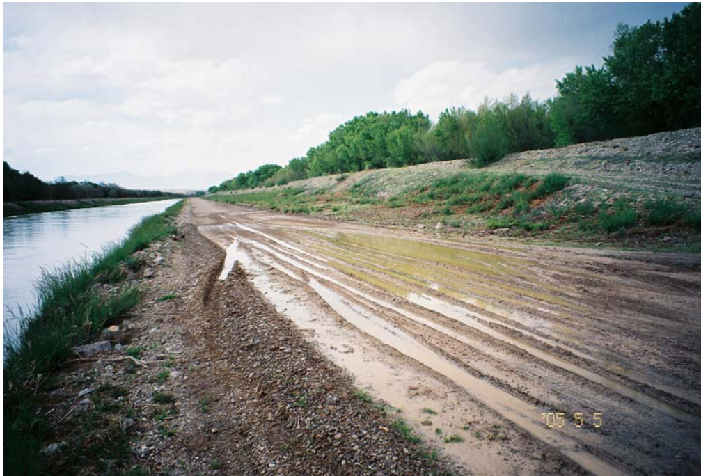
Photo 26: San Marcial Levee looking upstream near EB 12 showing accumulated seepage through the levee, LFCC on left and river behind levee on right (2005)
