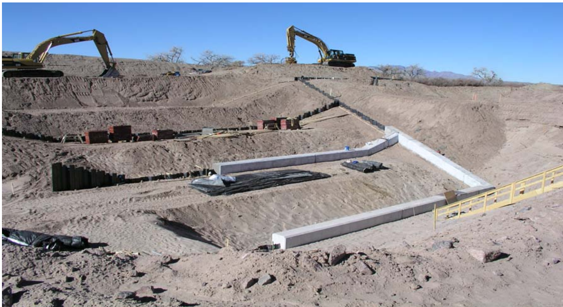
Photo 18: Photo taken 12-30-05, showing Contractor placing concrete grade control structure for San Lorenzo Arroyo. Four rows of sheet piles at 6-foot drops are shown. Photo taken by Cord Everetts.
