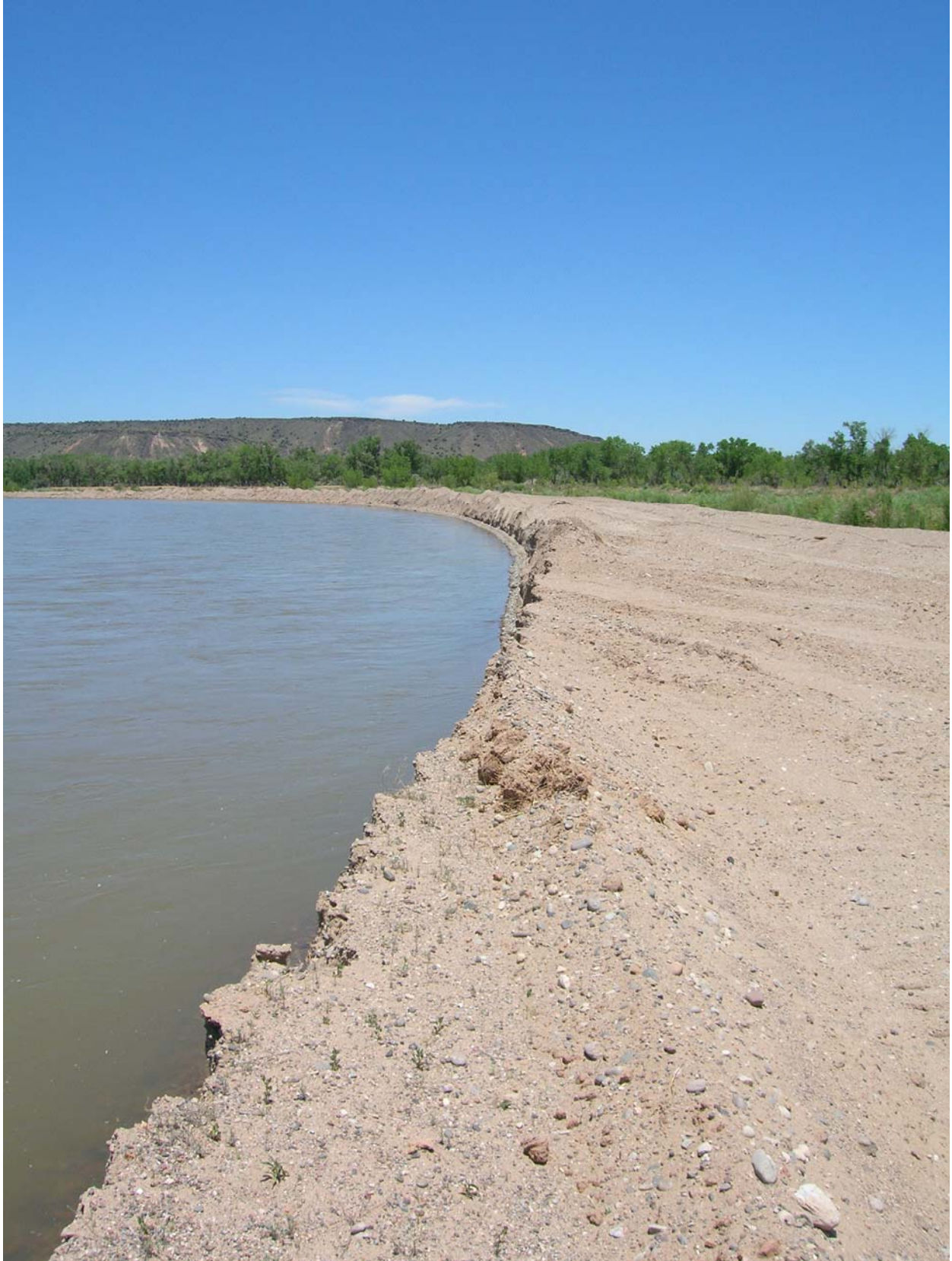
Photo 12: Erosion of excess sediment at Santa Ana, June 2005
