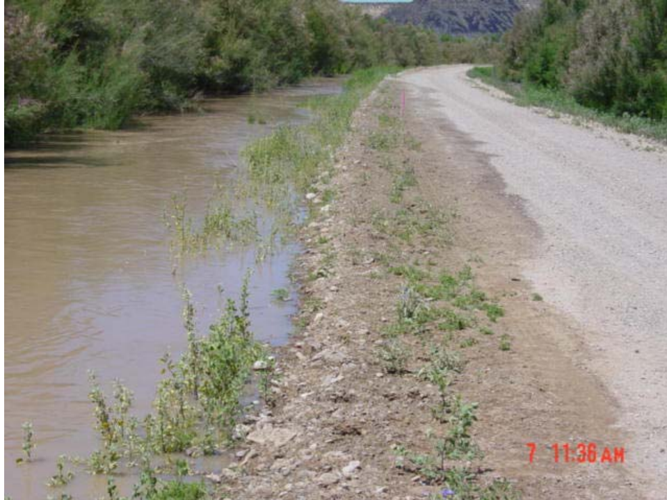
Photo 23: Tiffany Levee looking downstream at top of levee during spring runoff high flows with sediment plug in the river channel. Note that levee has no freeboard and is close to overtopping. (2005)
