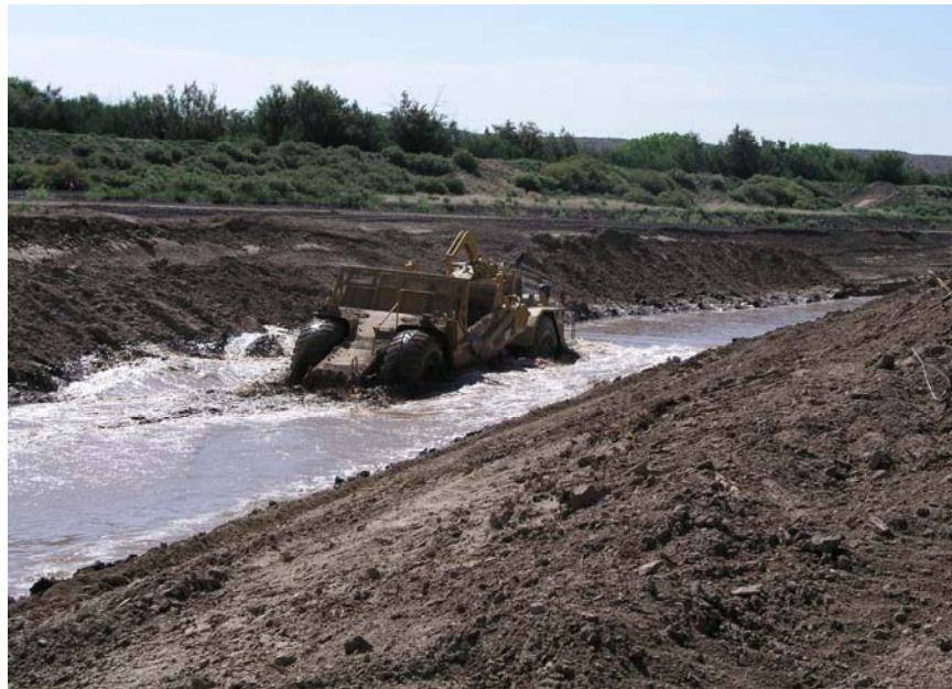
Photo 16: Photo taken 05-23-05, looking south (downstream) of station 1888+00. Photo shows a Cat 631 Scraper excavating material from the invert of new Low Flow Conveyance Channel. Groundwater is seeping into conveyance channel. Photo taken by Rudy Bernal, Bureau of Reclamation
