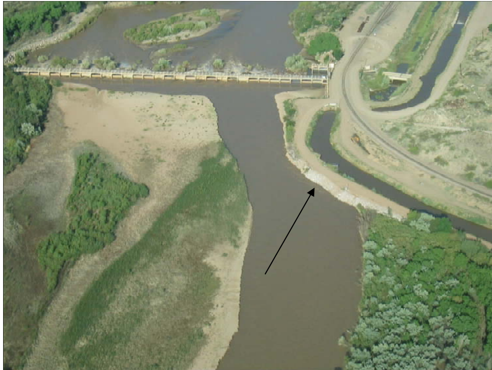
Photo 22: Drain Unit 7 immediately upstream of San Acacia Diversion Dam, arrow identifies location requiring riprap protection during spring runoff high flows (2005)
