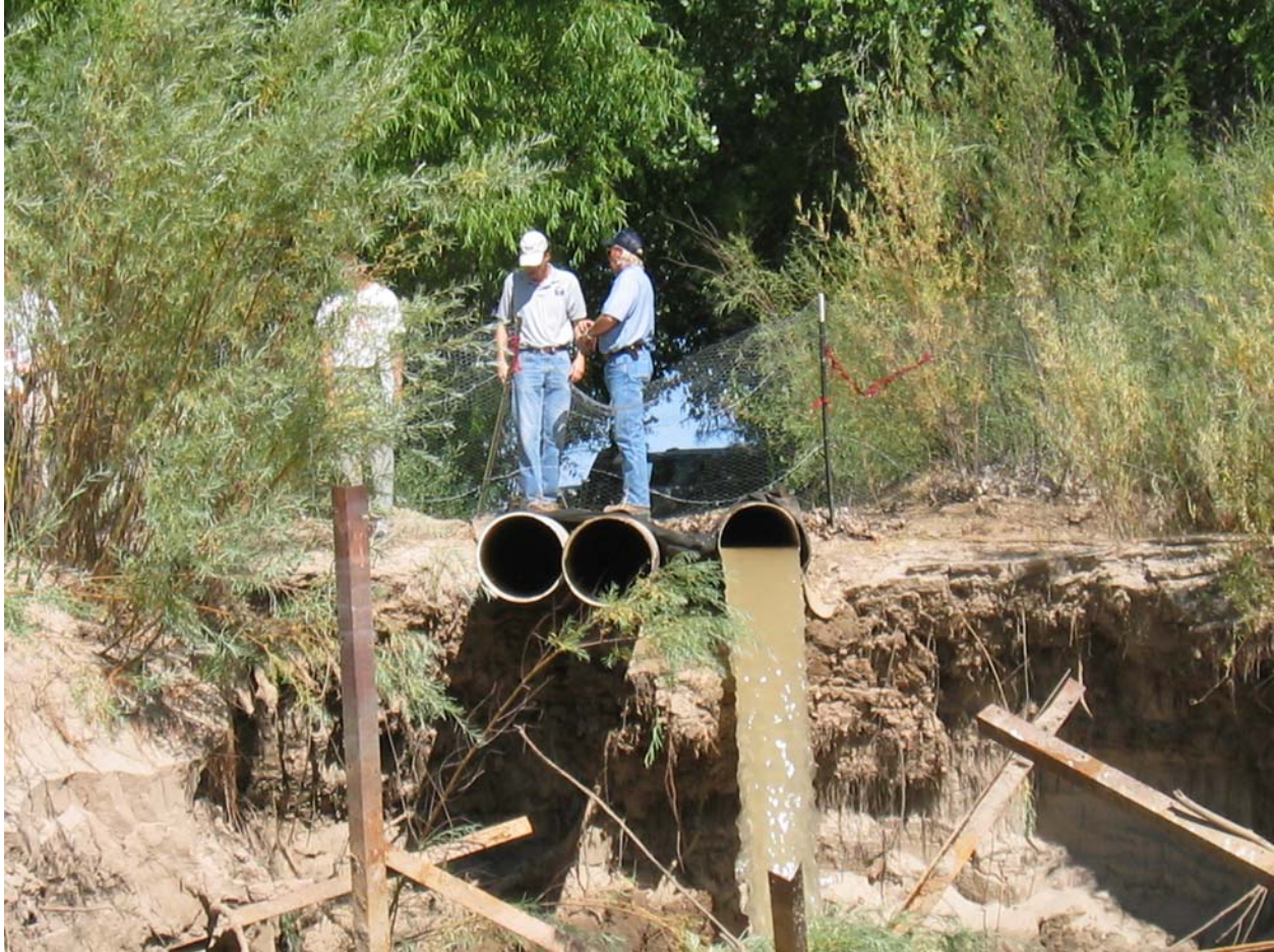
Photo 30: Post Runoff review at the Ft. Craig pump site location looking at west bank showing bank erosion and increased bank height from channel degradation (July 2005)
