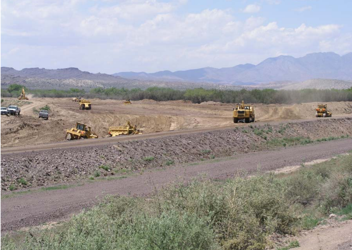
Photo 15: Photo taken on 05-16-05 at Station 1878+00. Shown are scrapers excavating for the new Low Flow Conveyance Channel. Photo taken by Rudy Bernal, Bureau of Reclamation.
