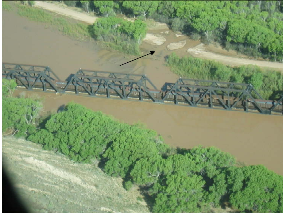
Photo 25: San Marcial Railroad Bridge crossing during spring runoff looking downstream. Arrow denotes breaches that occurred along the interior berm. (2005)
