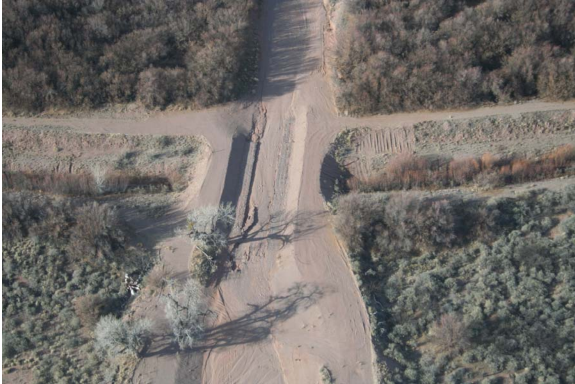
Photo 3. Completed Phase I work on Escondida Drain at Arroyo de los Pinos. Taken facing east (January 2008).
