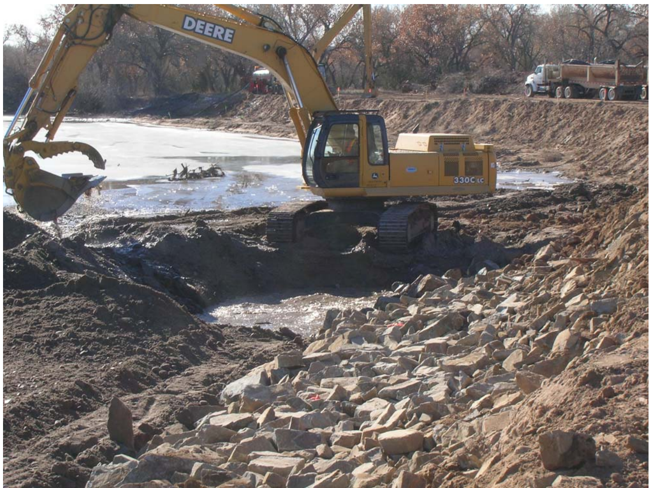
Photo 5. Installation of a riprap toe on the bankline at River Mile 231.3 (January 2008).
