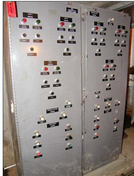
Photo 33 - Penstock control cabinet.
