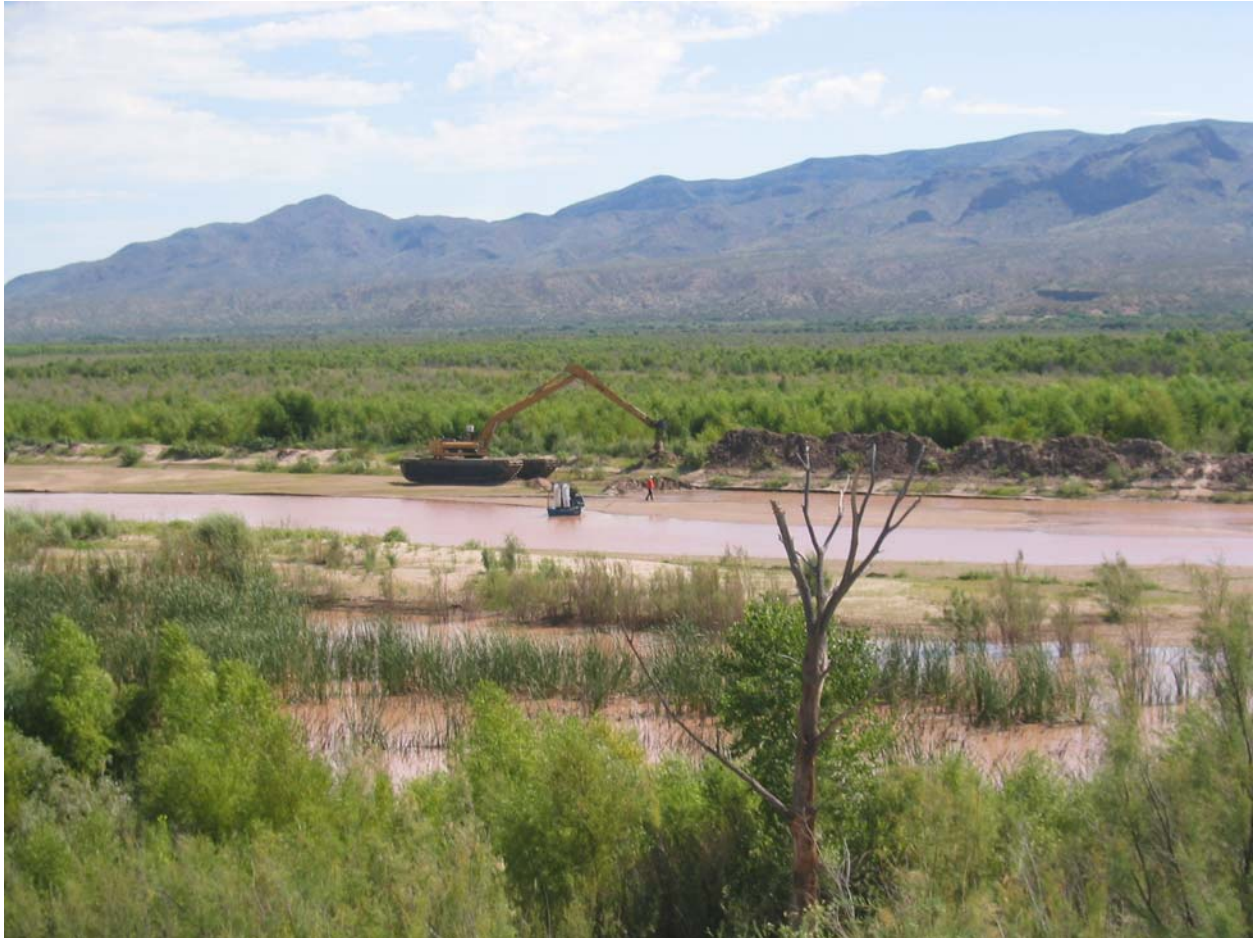
Photo 6. Amphibious excavator working on pilot channel through Temporary Channel sediment plug (September 2008, Weems).
