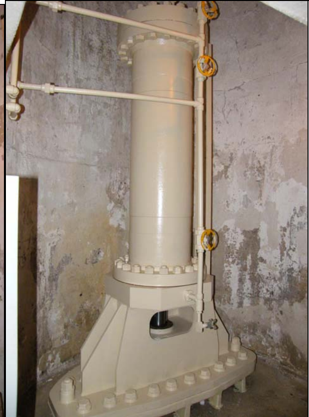
Photo 31 - New penstock gate operator - hydraulically operated.
