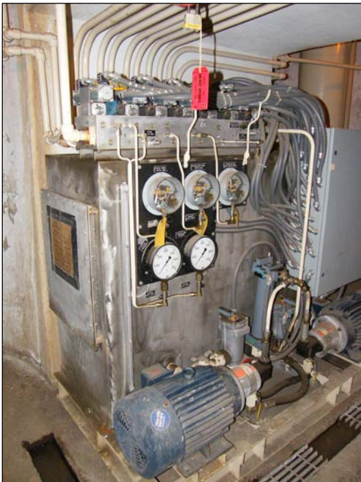
Photo 32 - Hydraulic Pump manifold.
