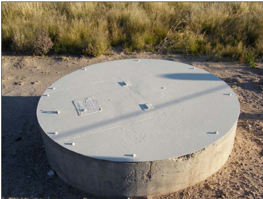
Photo 36 - Modified manhole showing new access hatch.
