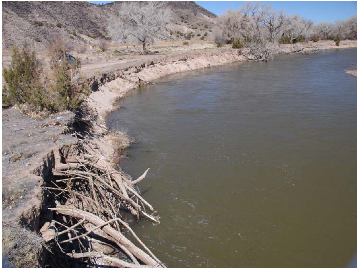
Photo 13. Upstream view of eroding terrace at Priority Site 213.4R, San Felipe. Note the location of the levee about 60 feet west of the bank edge. (February 2008, Mussetter Engineering, Inc.)
