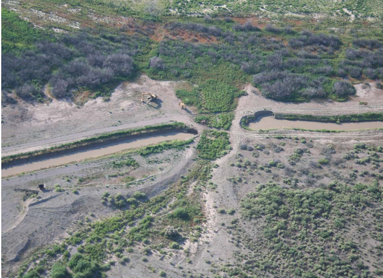
Photo 8. Collapsed culvert on Elmendorf Drain, looking east (July 2008, Gonzales).
