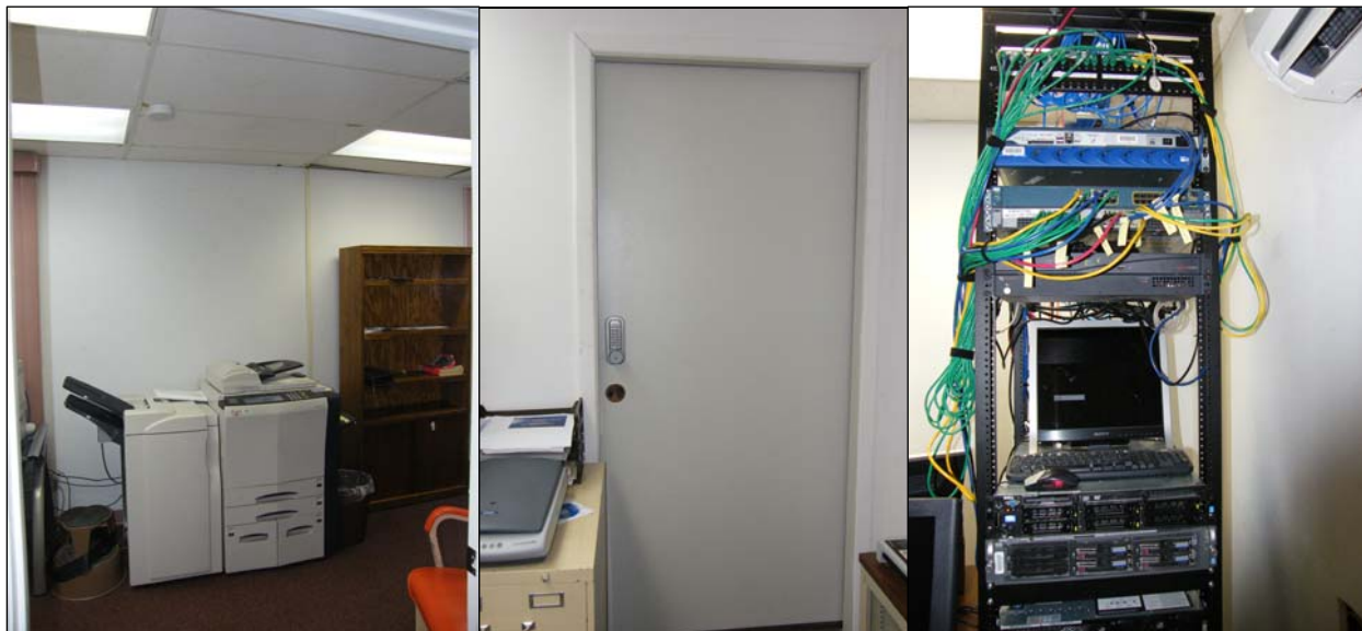
Photo 28 - Pictures showing old server location, new door access to server room, and the new servers on the racks up and running.
