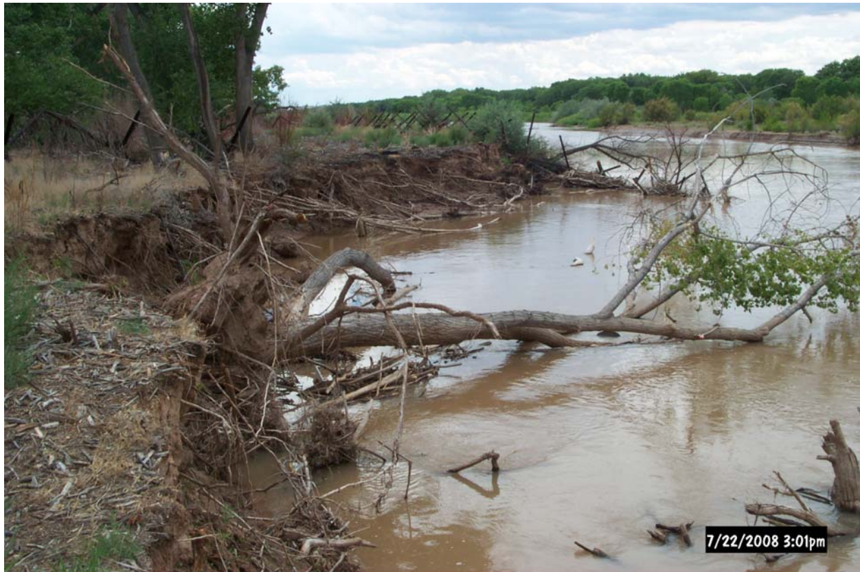
Photo 16. Looking downstream at the bend erosion at the Santa Ana Tamaya site (July 2008, AuBuchon)
