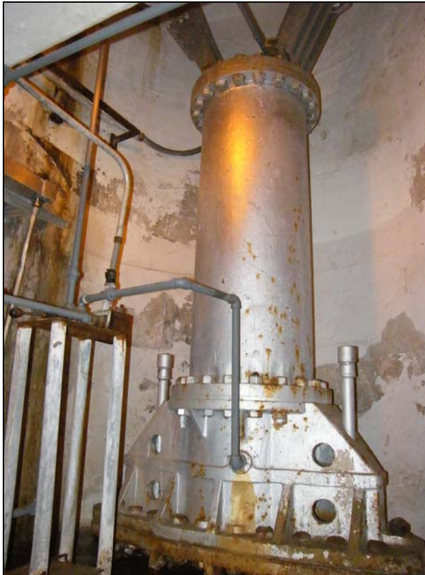
Photo 30 - Old penstock gate operator – water operated.
