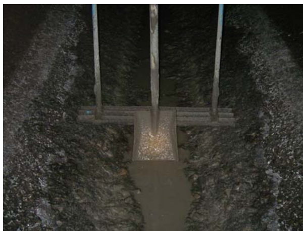
Photo 1. Azotea Tunnel prior to repair
