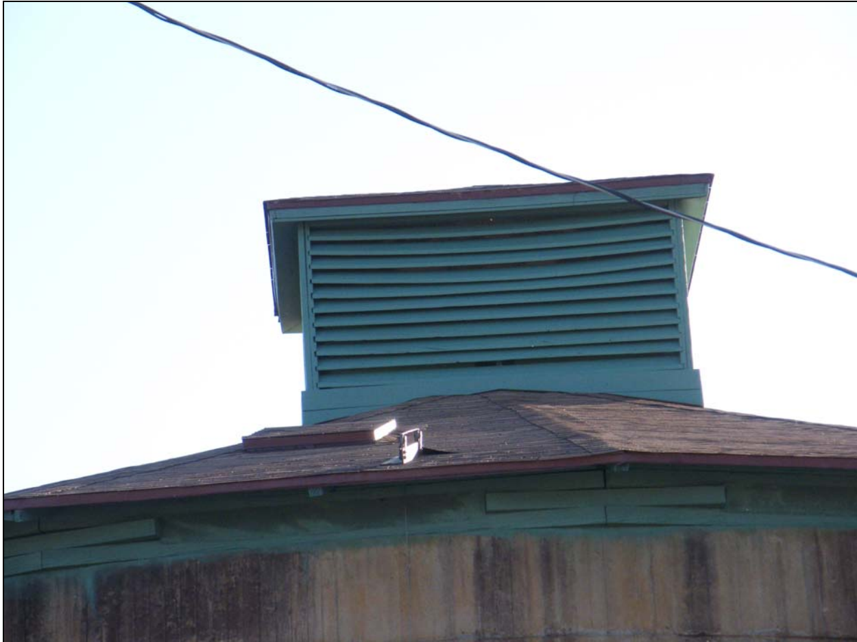
Photo 29 - Showing repainted vent box and redone roof as well as new access hatch.
