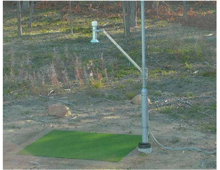
Figure 4: Sodankylä, angled mounting beam on 70:32
