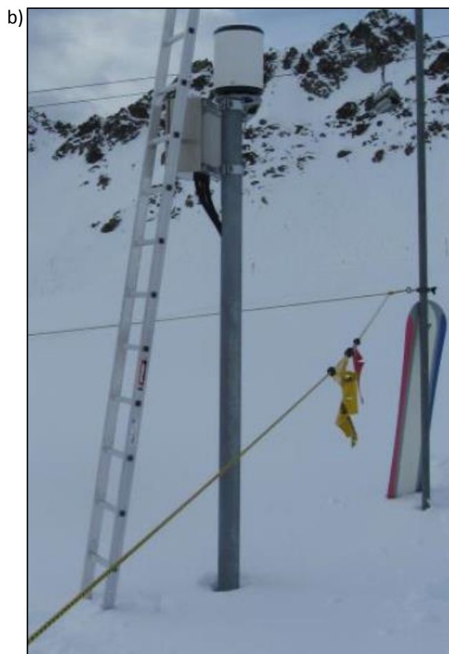
Figure 1: ZAMG MR3H-FC installations at (a) CARE and (b) Weissfluhjoch.
