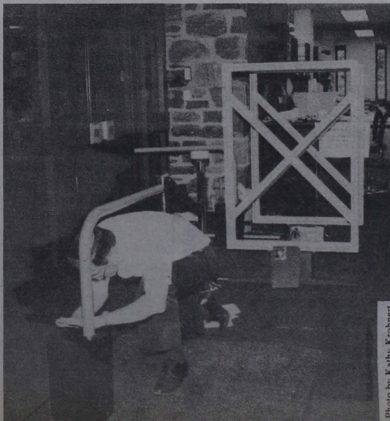
Myrin has detection system installed.
