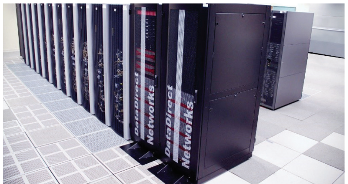
OHIO SUPERCOMPUTER CENTER
