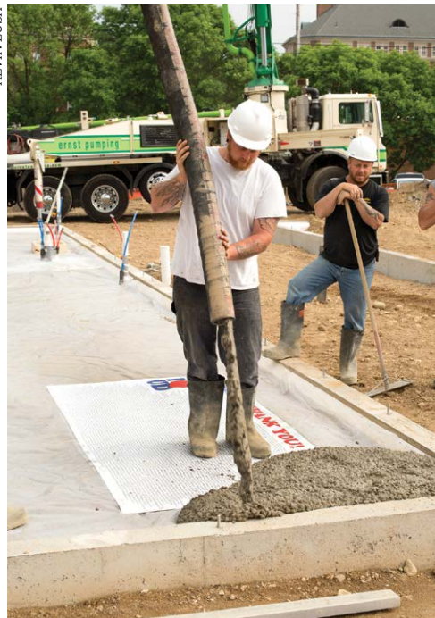
A construction worker pours cement over the banner that lists more than 800 donor names that became part of the foundation of the "I Love UD" house.
