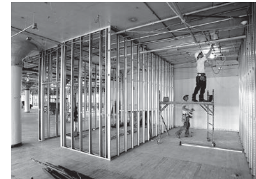
Workers begin renovations on the fourth floor of the College Park Center.
