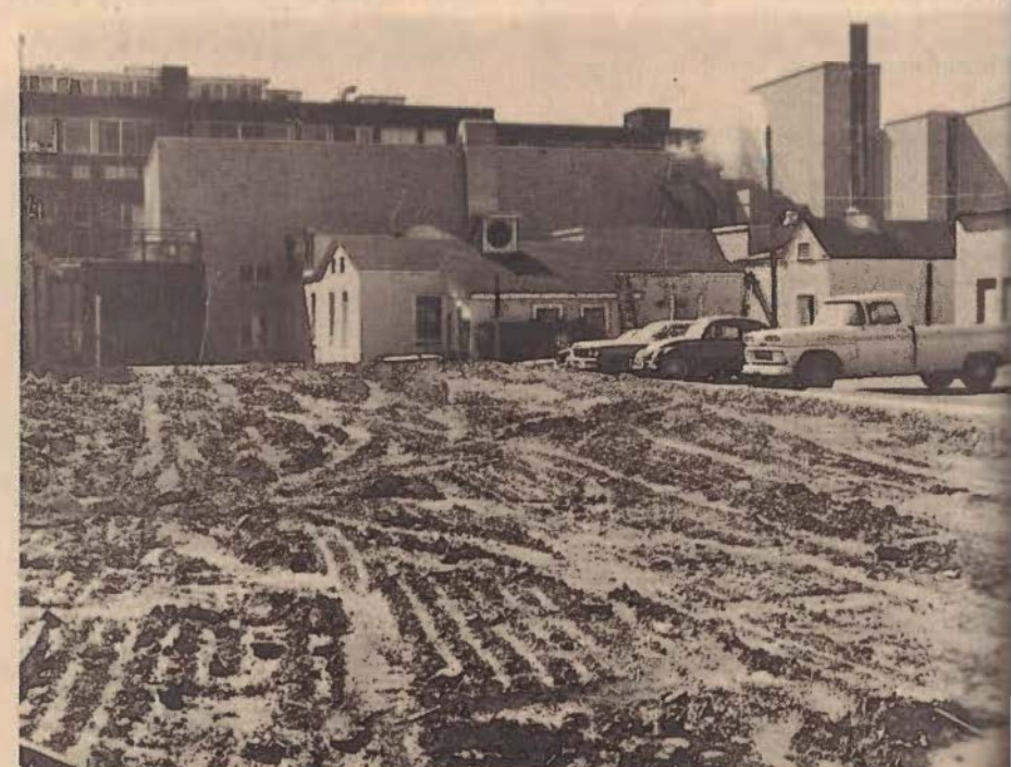
The Heims Building, which formerly occupied this spot, was torn down to make room for the new laundry. In the background is the old laundry which will be used as a store when the new laundry is built.
