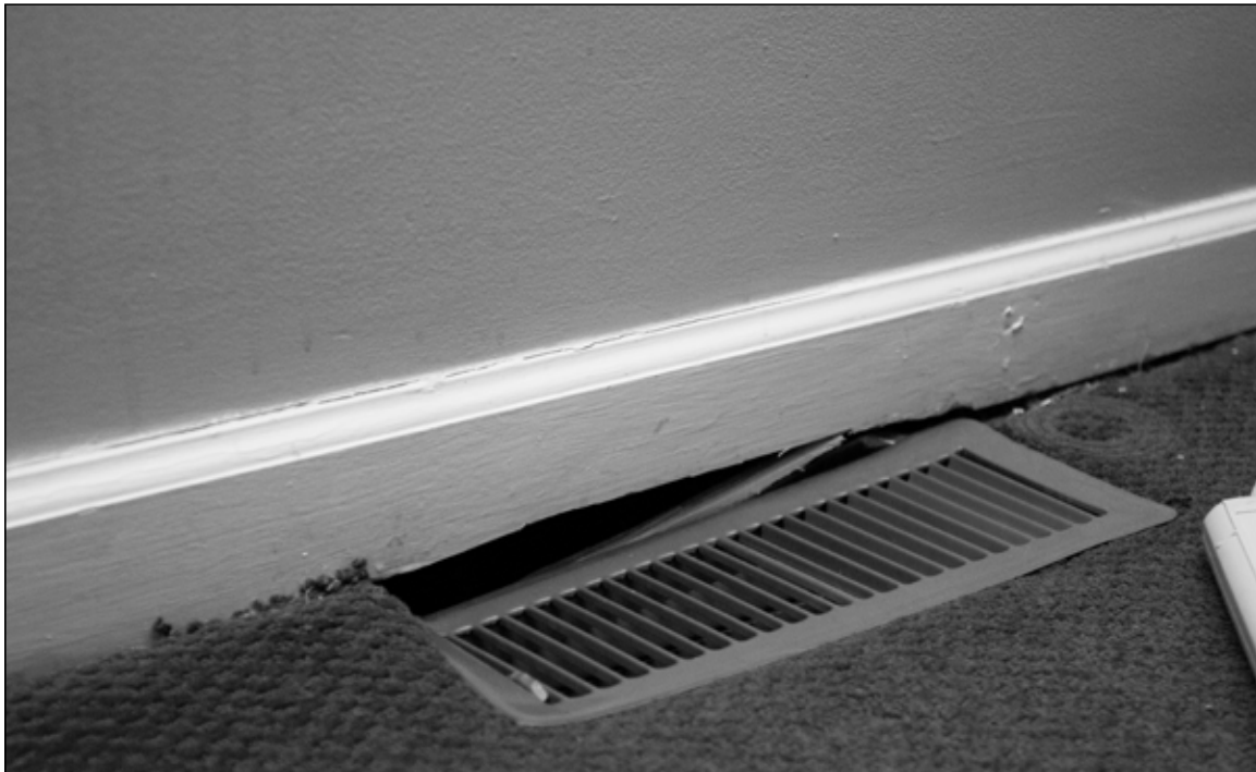
The partially collapsed floor inside a University of Dayton-owned residence at 218 Kiefaber Street is seen, Tuesday, Jan. 22. ETHAN KLOSTERMAN/MANAGING EDITOR
