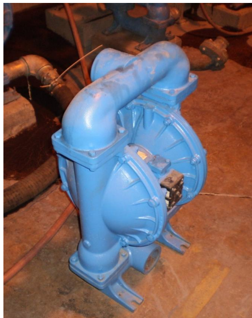
Figure 2. Air pumps use seven times more electricity than electrical pumps
