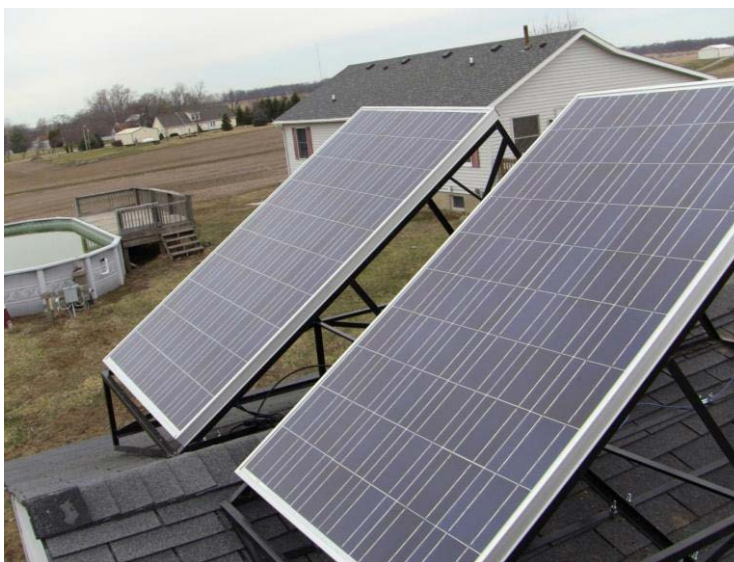
Figure 28: Solar panels used in solar irrigation system.
