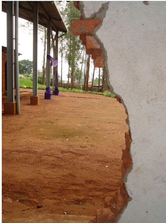
Figure 4A and 4B: Damage from grenade attack.
