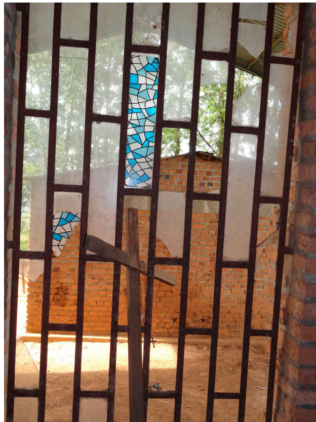
Figure 1A: The protective roof over the church. Figure 1B: Broken stained glass windows from the massacre.
