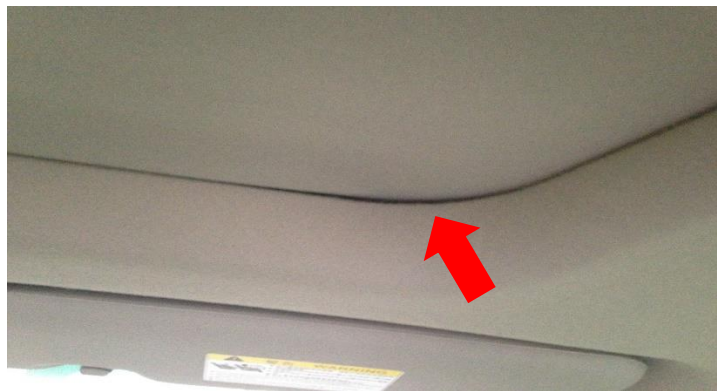
Figure 4: Gap between Skylight and Plafond
