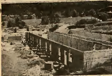
Construction of the new dorm addition to Thatcher Hall has begun. (Photo by Sharon Webster).
