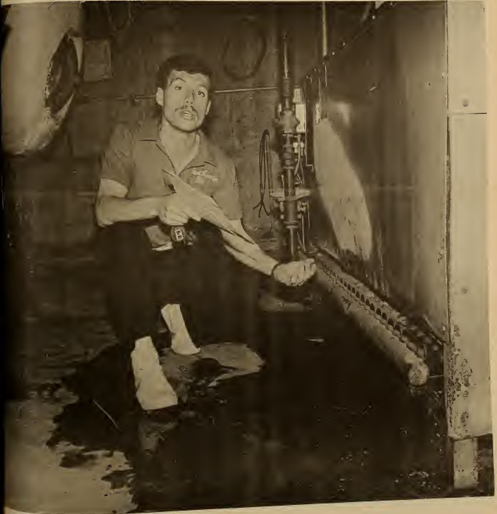
Hot Water Up in Flames
