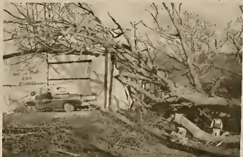
Did it get too old to hold itself up anymore, or did the recent weather do it in? Either way, the Emergency Medical Services building on Ooltewah-Ringgold Road won't be in use for quite some time.
