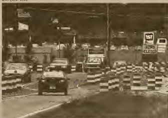
Overdue: Motorists pass through the Apison Pike construction area as it draws to a close after more than a year.
