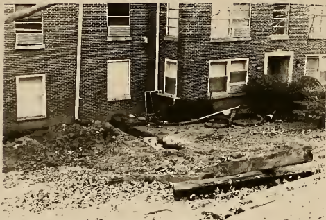
What a Mess! The digging that has been taking place around campus is for fiber optic cables that will be used to upgrade the communications system. Talge Hall, above, is one of the buildings that will benefit from the new cables.
