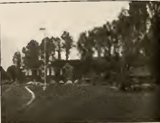
Builders break ground in Southern Village preparing for the construction of more buildings and parking.
