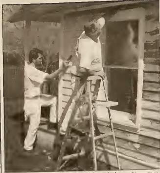
University painters Eddic Galera and Roger Anderson chip away at old layers of paint on the historic Doll House. The oldest structure on campus, it was built by James Thatcher in 1906 for his daughter. It has been used as a library, president's office, shoe repair shop, prayer room, storage for bee hives and a WSMC microwave relay station. It was restored in 1981 and is now getting a fresh coat of paint.
