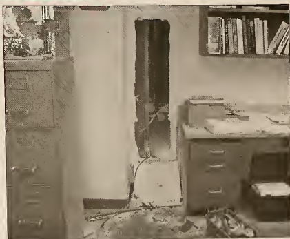
Most of the visible damage in Keith Snyder's office came from the fire department cutting a hole in the wall to get to the burned insulation.
