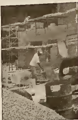
Renovating Hackman Hall is just one of the projects Advancement is working on.
