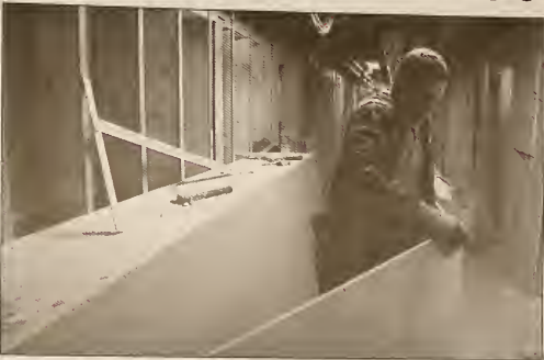
Dan Ford, Plant Services foreman, continues with the construction on Lynn Wood Hall. The renovation has been going on since the spring of 2004.
