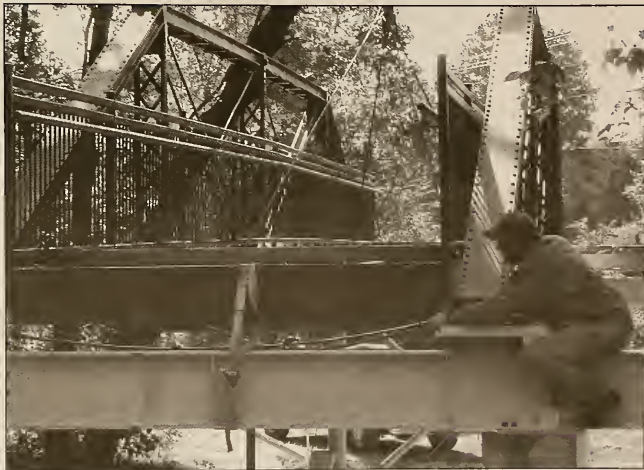
Jeff Sparks connects the new Greenway bridge on High Street Friday morning.
