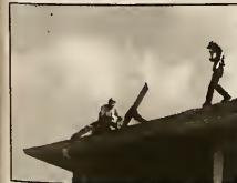
Photo by Sonya Reeves Above All Roofing employees repair the fire-damaged shingles on the roof of Lynn Wood Hall Tuesday afternoon.
