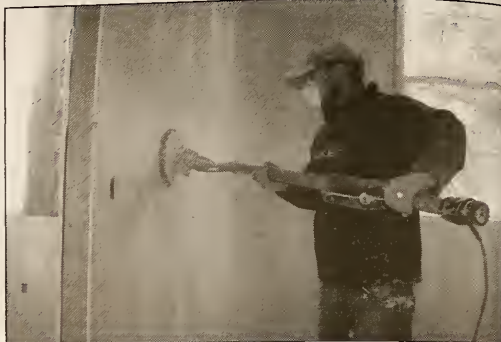
Tennessee Drywall Company employee Joe Wenz blasts the second floor wall in Lynn Wood Hall Wednesday afternoon. The completion date for Lynn Wood Hall is set for August.
