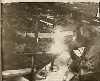
Paul Sabo welds a set of stairs by Daniel's that leads to the new parking lot on Industrial Drive Monday afternoon.
