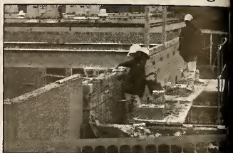
File Photo by Rebecca Burkhart Kuehler Builders work on the new building for Collegedale Academy as they are building a new science facility.
