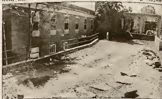
Photo by Devin Page Future location of Kelly's Garden, currently under construction.
