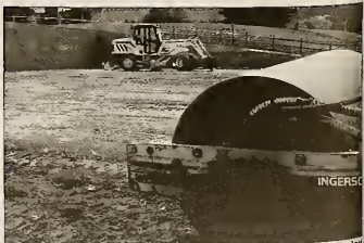
Construction equipment readies the ground for the new tennis courts behind Iles P.E. Center. Photo by Matt Barclay
