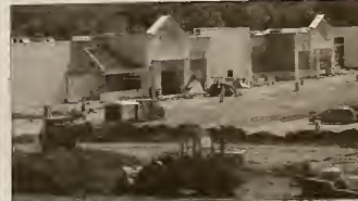
Construction on the Collegedale Wal-Mart continues. The store is expected to open the beginning of 2007.
