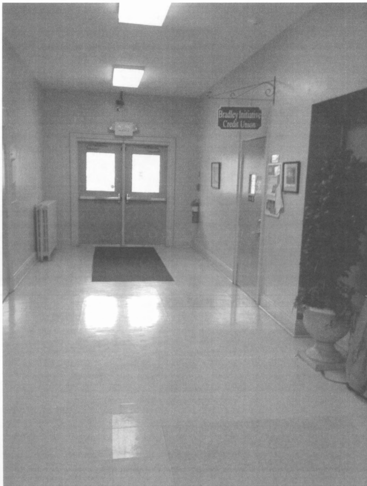
Fire Extinguisher @ Opposite End – West Doors
