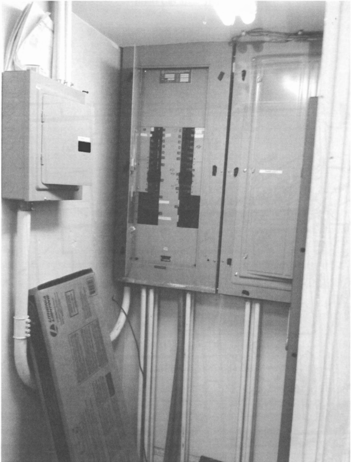
Breaker Boxes inside Suite 12 Left-hand Closet
