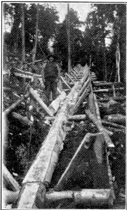
Fig. 13. A pole chute under construction. All of the substructure was erected previous to the installation of the trough. Eastern Canada.
