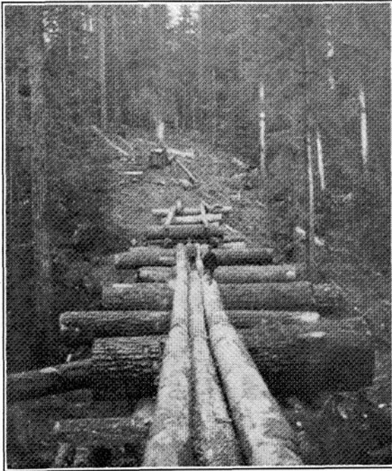
Fig. 27. A "fore-and-aft" road under construction. The heavy cribwork in the foreground serves to carry the channel over a deep depression. The construction timber is brought into place by the donkey engine shown in the background. Oregon.
